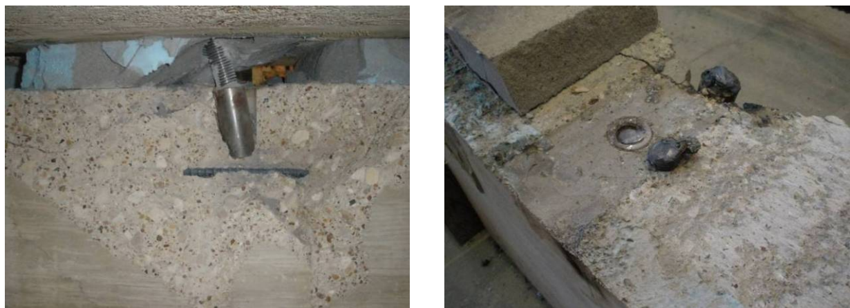
Figure 3-30. After Exhibiting Sliding Shear past 1.0 in. (25 mm) Relative Displacement, One of the Threaded Rods in 2_TRC_2.0_A Sheared at the Top of the Coupler and the Beam Cover Concrete Spalled off as the Load Was Redistributed to the Other Connector.
