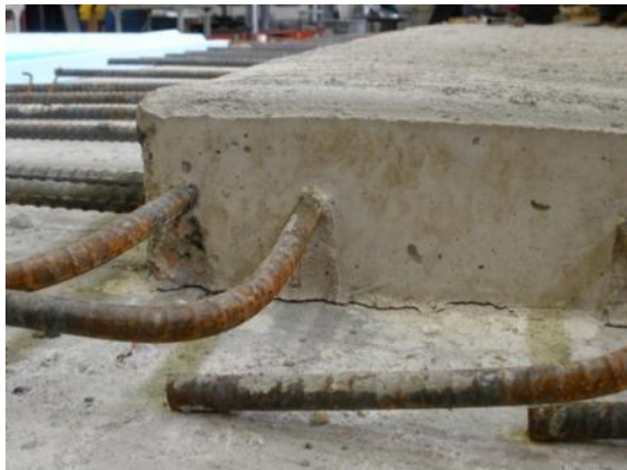
(a) Cracking between Stage I and II
