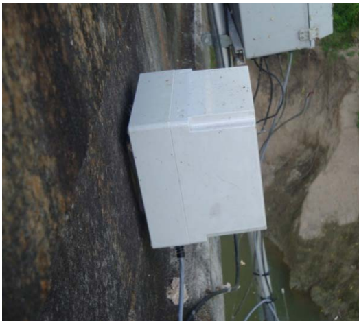
Figure D-13. Single-Axis Tiltmeter 1 on the Deck Adjacent to Master Station at Pier SB2.
