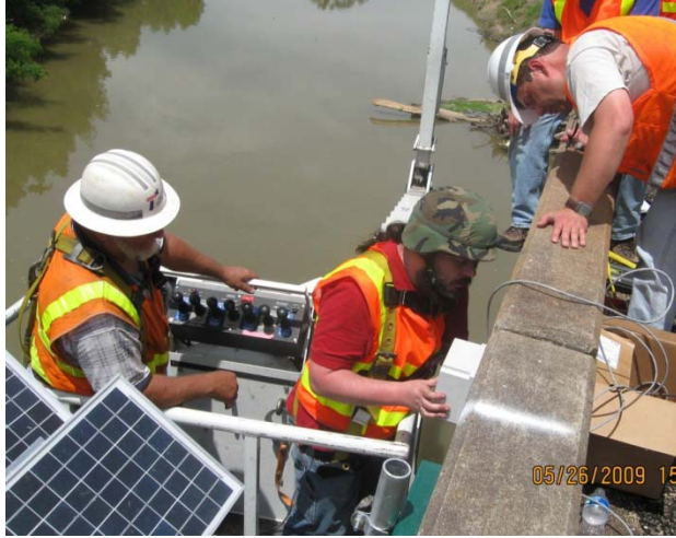
Figure D-9. Positioning the Tiltmeter.
