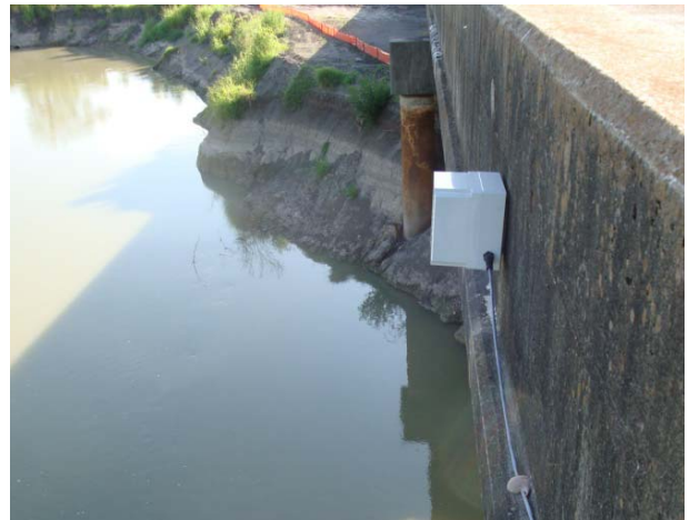
Figure D-14. Single-Axis Tiltmeter 2 on the Deck at Pier SB1.
