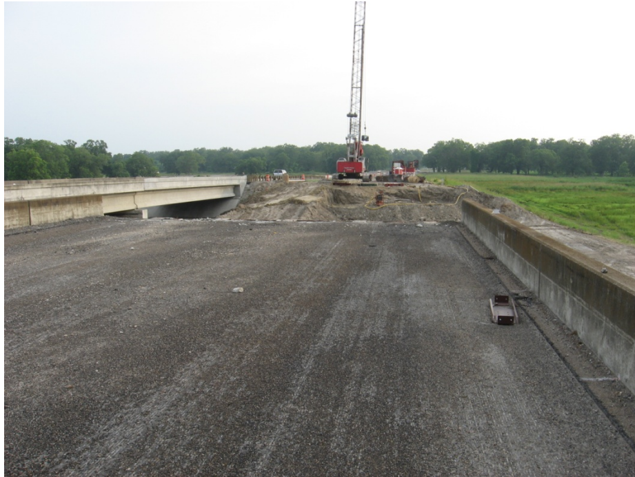
Figure 5-4. Construction on the Extension of the Southbound Lane of US59 over Guadalupe River Bridge.
