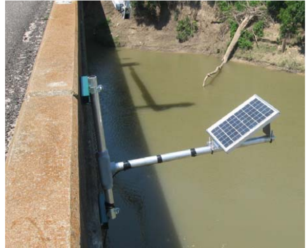
Figure 5-12. Solar Panel on the Pier SB1.
