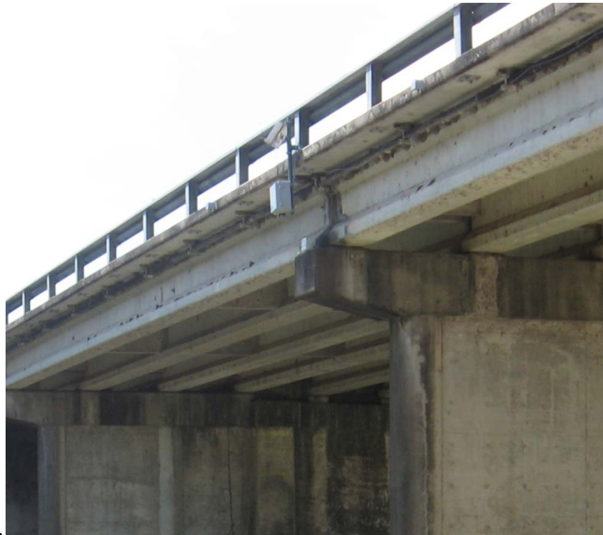
Figure E-16. Bridge Scour Monitoring System.
