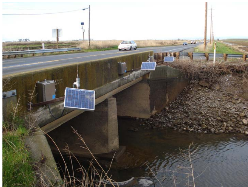
Figure C-8. Tiltmeter Installation (Caltran).
