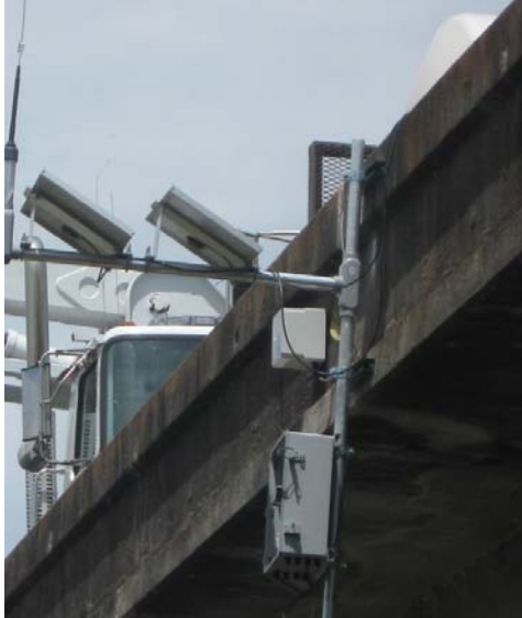
Figure 5-9. Installed Dual-Axis Tiltmeter.
