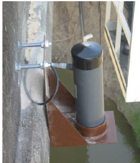
Figure 5-10. Installed Water Stage Sensor.
