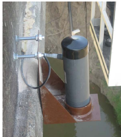
Figure D-18. Installed Water Stage Sensor.
