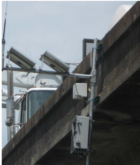
Figure D-11. The Installed Tiltmeter, Master Station, and Solar Panels.
