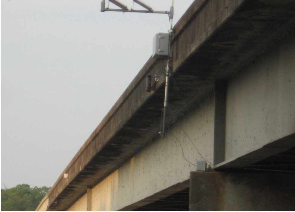
Figure D-15. Bridge Scour Monitoring System (View from South Side of the Bridge).
