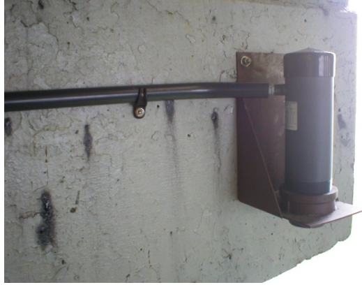
Figure C-13. Water Stage Sensor Mounted on Pier Cap (NYSDOT).
