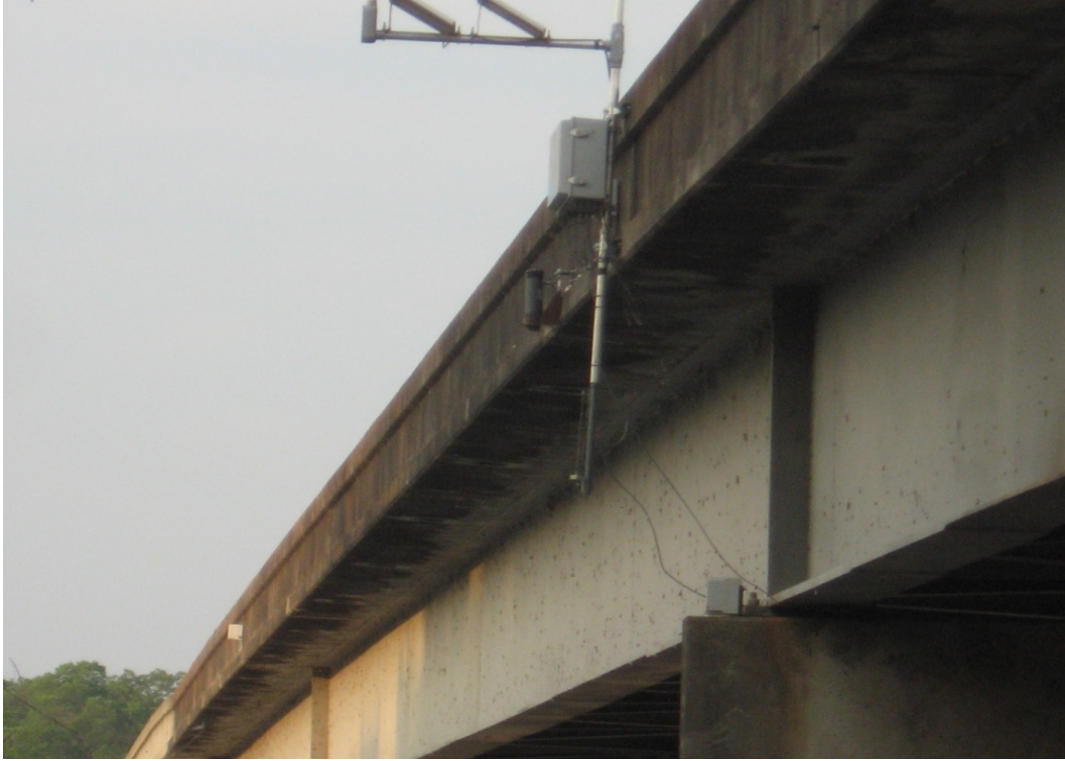
Figure 5-28. Modified Bridge Scour Monitoring System.
