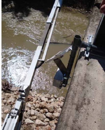
Figure 6-15. Solar Panel for the Accelerometer on the Cap Beam of Pier P1.
