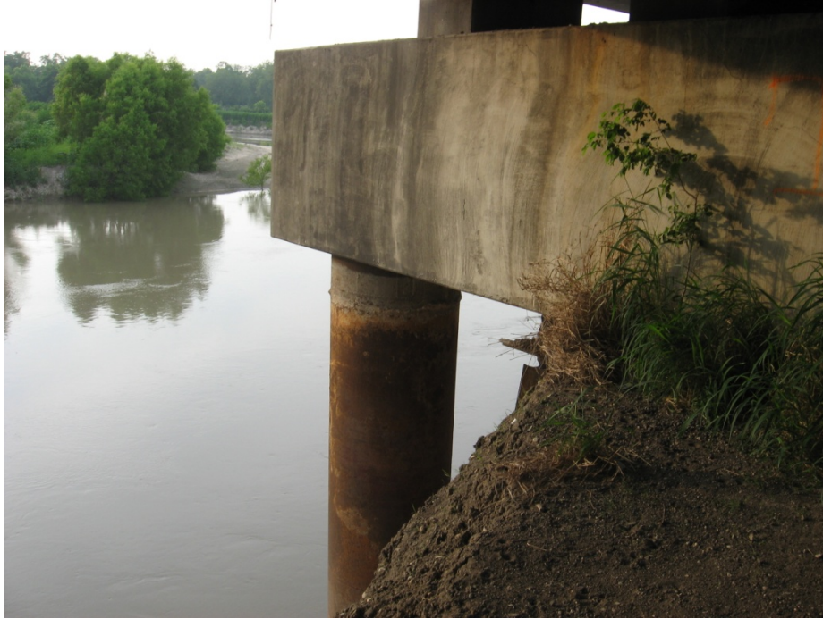
Figure 5-6. Drill Shaft on Northeast Side (SB0) of US59 over Guadalupe River Bridge in 2010.
