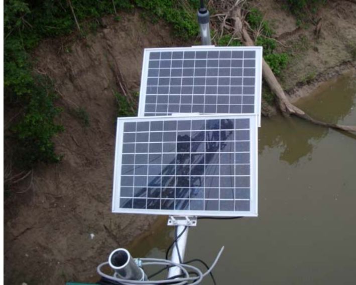
Figure 3-12. Solar Panel near the Data Acquisition System on the Bridge.
