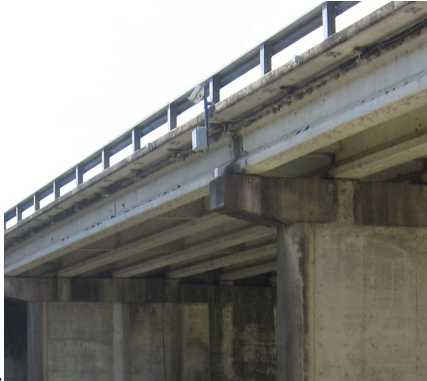
Figure 6-20. Modified Bridge Scour Monitoring System.
