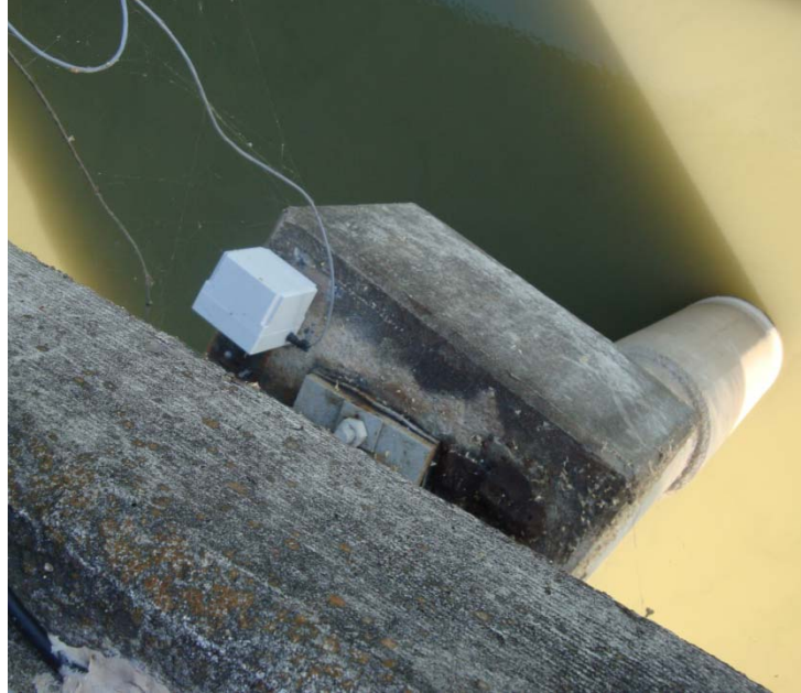
Figure D-12. Dual-Axis Tiltmeter on the Pier SB2.
