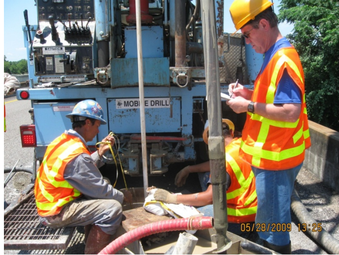
Figure D-26. Refilling the Drilled Hole after the Installation of the Float-Out Devices.
