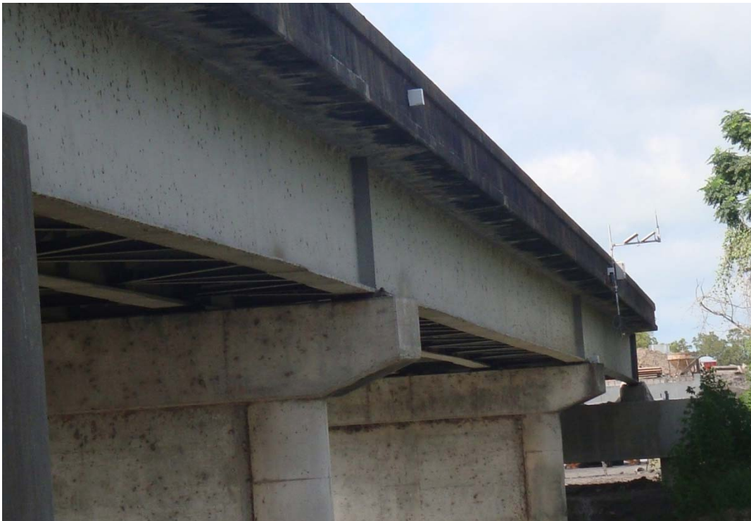
Figure D-16. Bridge Scour Monitoring System (View from North Side of the Bridge).
