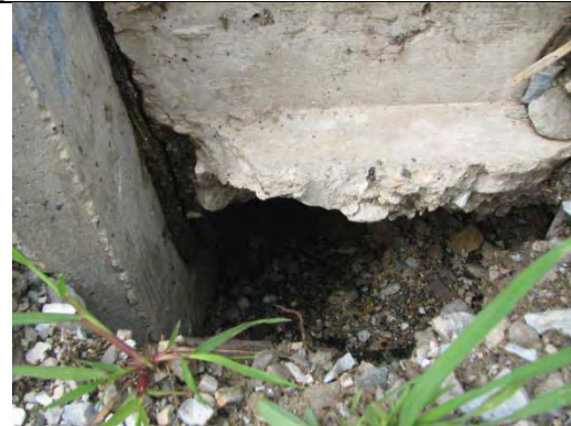
Erosion of soil underneath BAS
