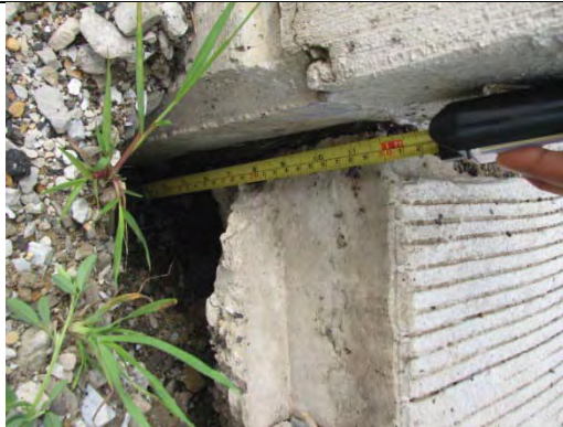
Erosion of soil underneath BAS
