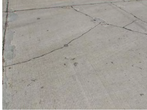
Surface cracking due to uneven settlement
