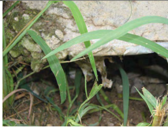
Erosion of soil underneath BAS
