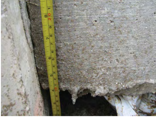
Soil erosion underneath BAS
