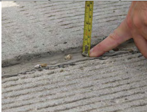
1/2" Bump at other end of the bridge
