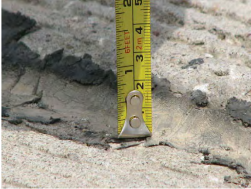
1" Bump at end of the bridge
