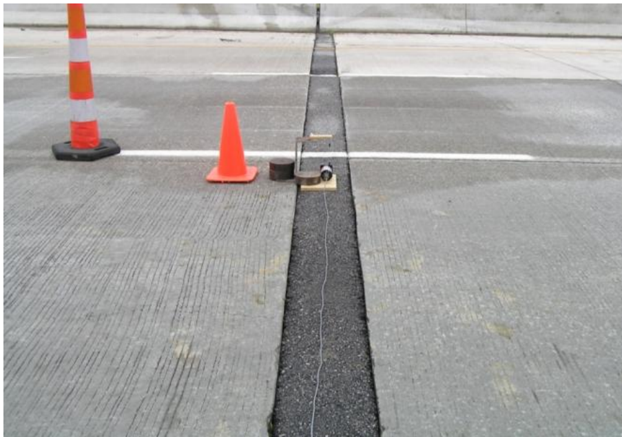
Figure 5.45. 12 in. pressure relief joint condition
