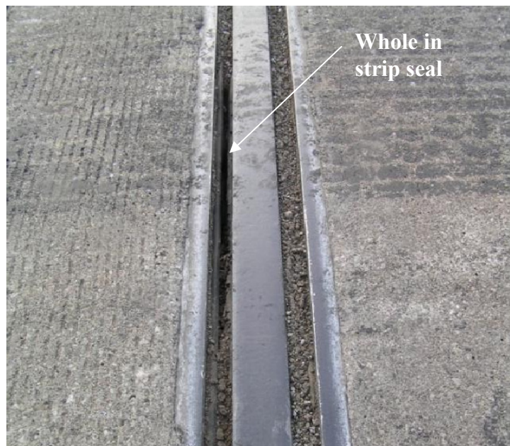
Figure 5.54. Deterioration of strip seal
