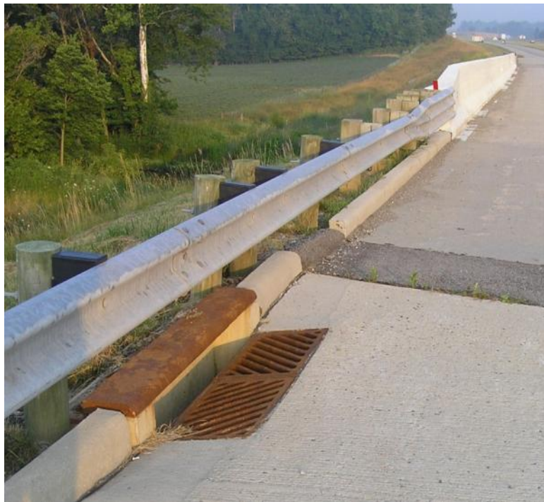
Figure 5.42. Bar grates and curb provide good water drainage and eliminates erosion at the edge of the shoulder
