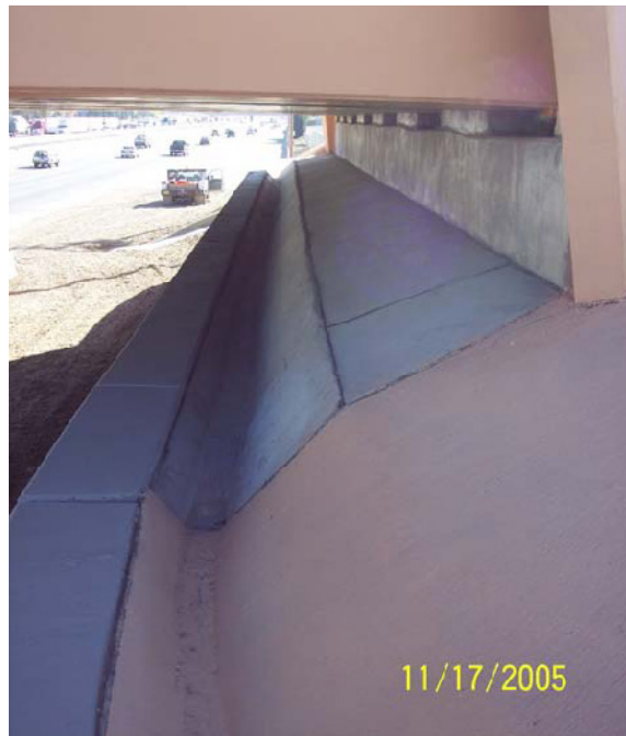
Figure 4.37. Drainage gutter used in New Mexico for moving water away from the bridge embankment (Lenke, 2006)
