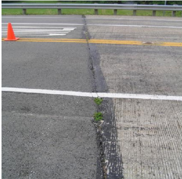
Figure 5.37. Pavement-to-approach joint condition at LIC 40-12.53
