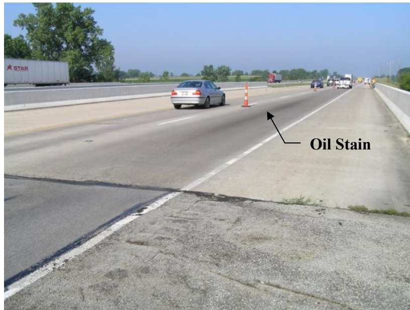
Figure 5.34. Oil staining on bridge surface caused by bump at pavement-to-approach joint
