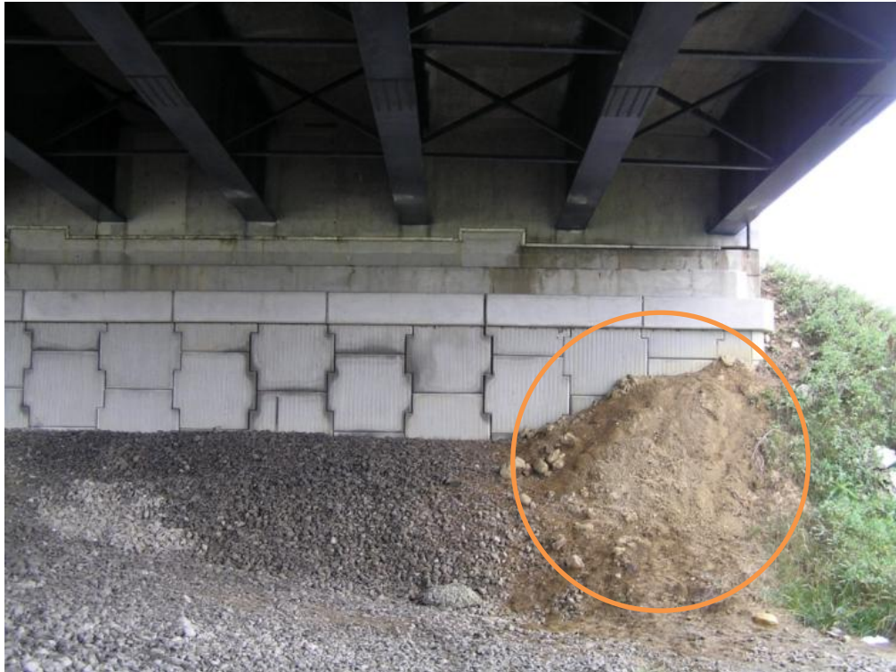
Figure 5.46. Erosion from bridge embankment
