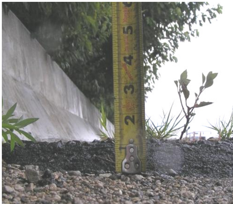
Figure 5.28. Differential settlement at pavement and bridge abutment
