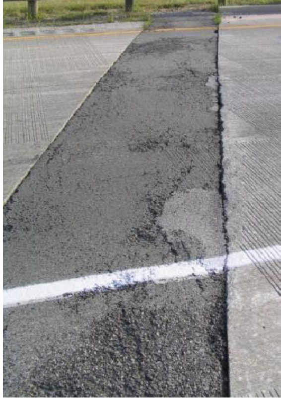
Figure 5.41. WYA 30-22.40 pressure relief joint deterioration
