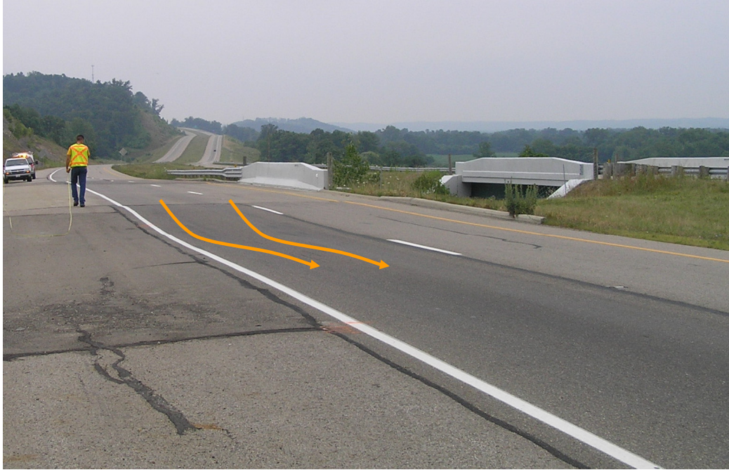
Figure 5.17 Dip in pavement when exiting the bridge
