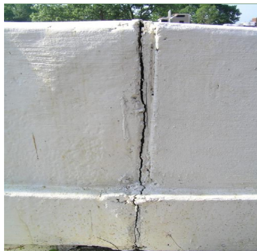
Figure 5.33. Barrier rail joint at approach slab showing settlement of approach slab
