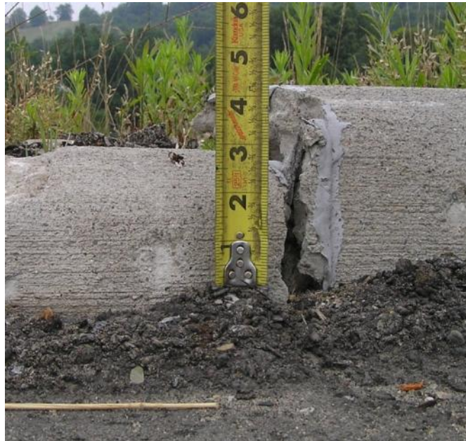
Figure 5.15. MUS 16-7.69 approach slab settlement relative to main line pavement
