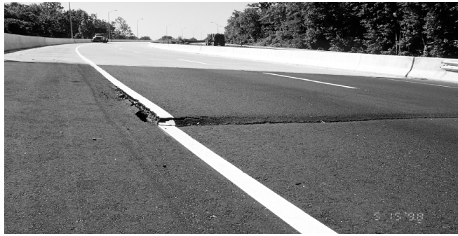
Figure 4.60. Approach slab distress attributable to foundation soil settlement (Route 10 westbound lane over the Appomattox River) (Hoppe, 1999)
