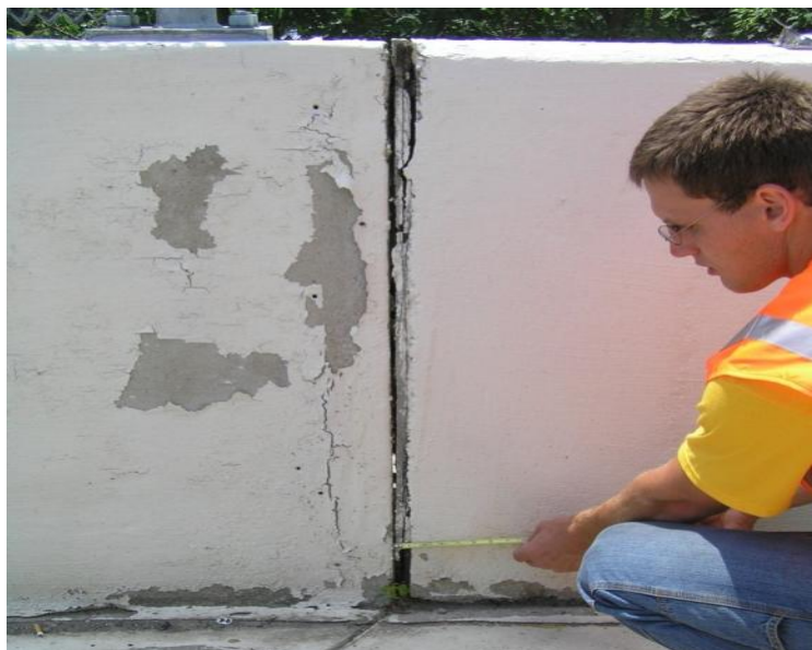
Figure 5.23. Tapered vertical gap at bridge to approach slab joint indicating settlement
