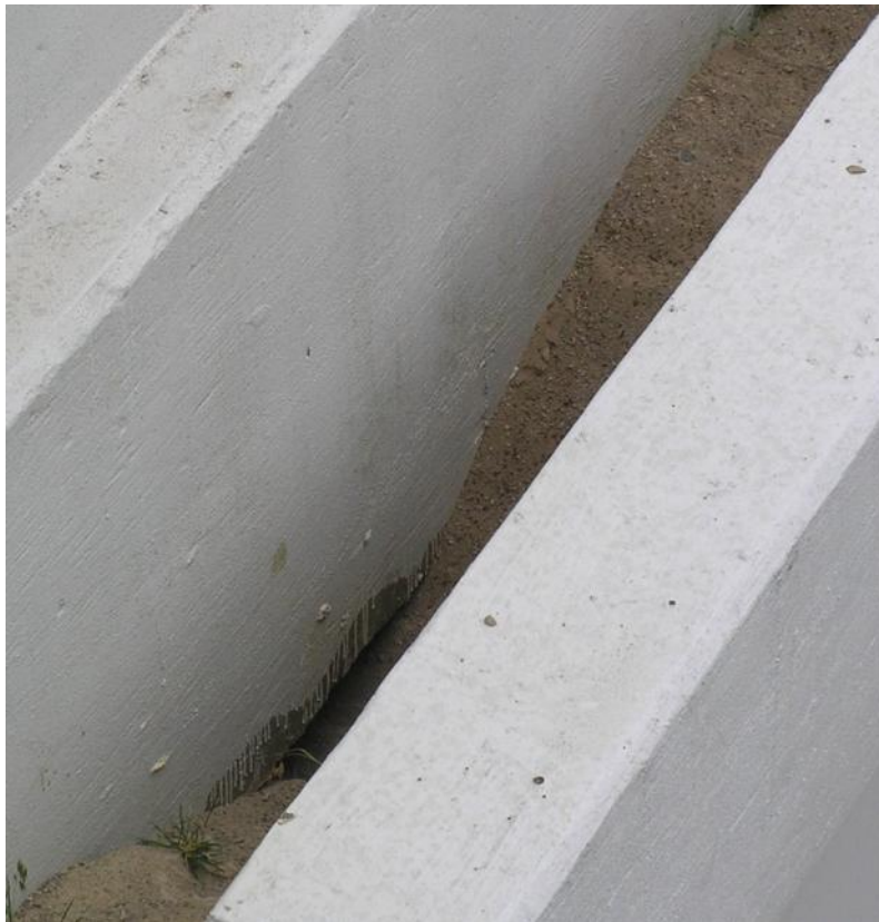
Figure 5.18. Fill loss between the MSE wall and the bridge abutment
