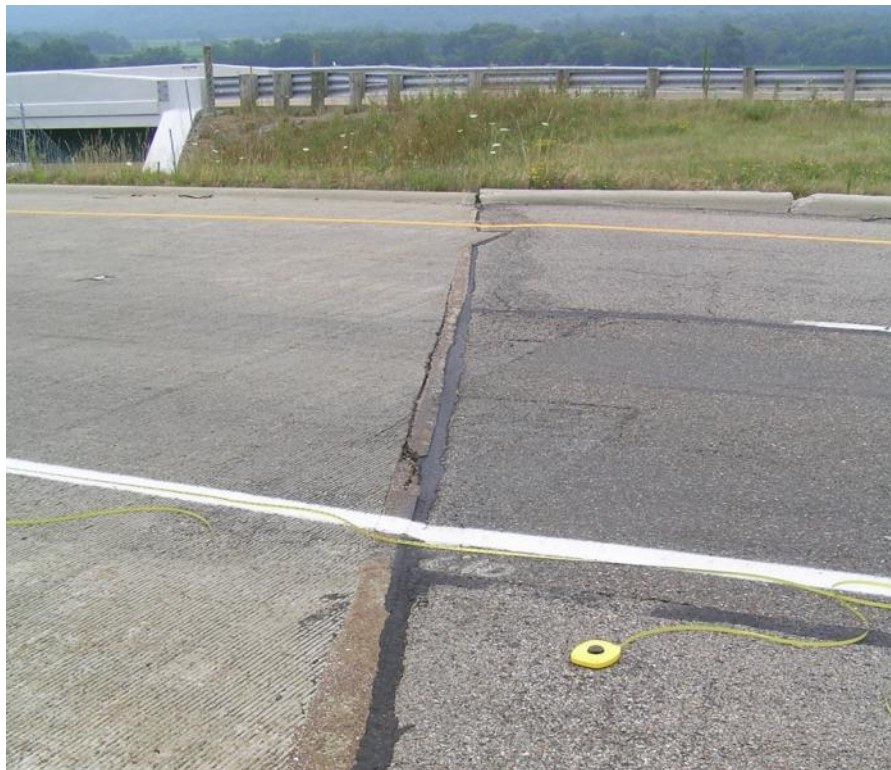
Figure 5.16. Approach to pavement joint filled with grout causing a hump
