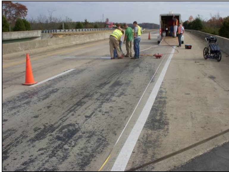
Figure 3-21: View of the bridge deck on the Courtland Bypass over Norfolk Southern RR
