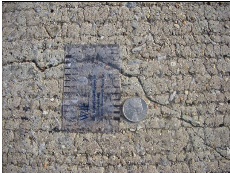
Figure 3-22: Picture of the wide surface cracks on the bridge deck on the Courtland Bypass
