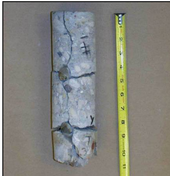
Figure 3-14: Core from CRC pavement in Texas with vertical and horizontal cracks (Courtesy of Dr. Moon Won)
