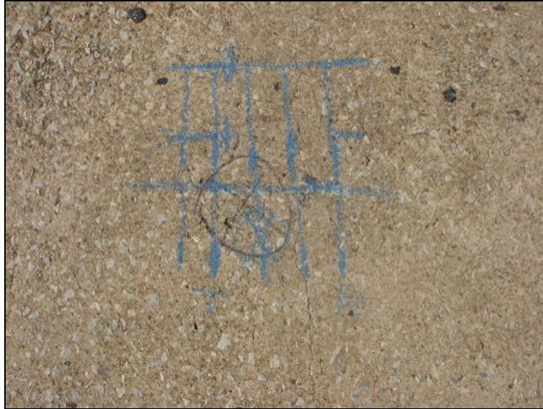
Figure 3-20: Pictures of the bridge deck on SR 49 over SCL RR in Lineville
