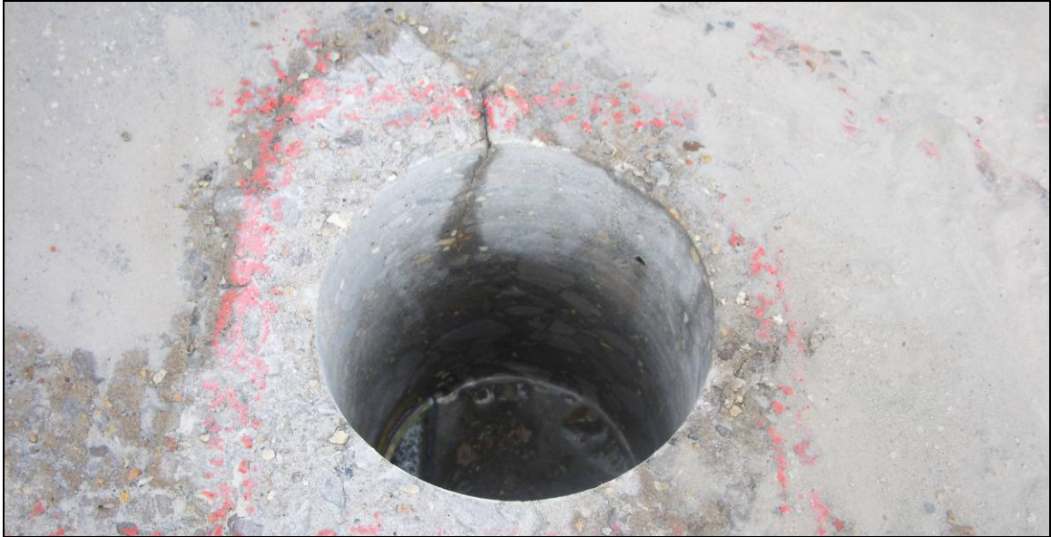
Figure 3-23: Pictures of the core hole on the bridge deck on the Courtland Bypass
