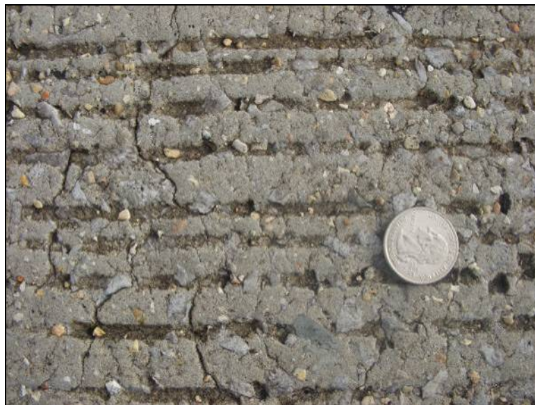
Figure 3-25: Picture of some surface cracks on the bridge deck on SR 216 over L&N RR
