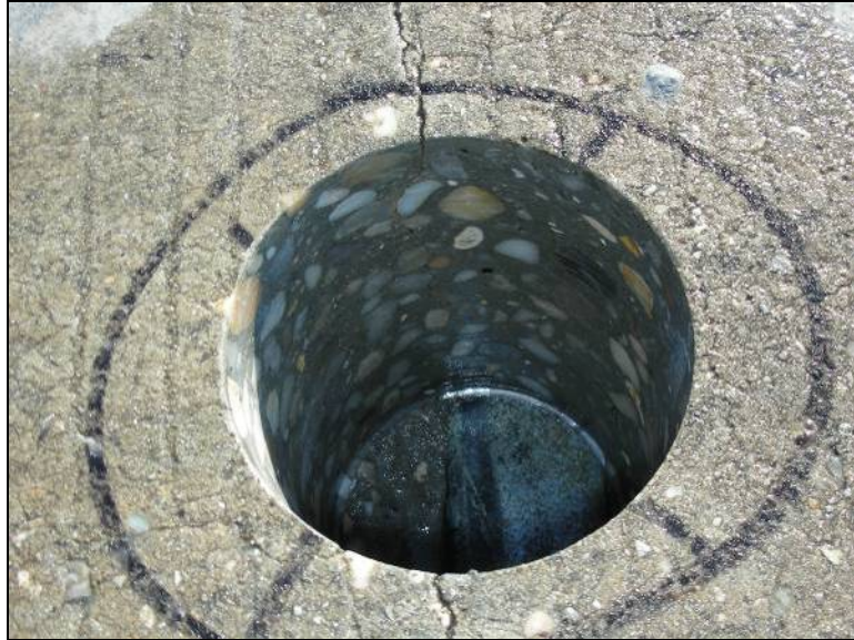
Figure 3-28: Picture of the core hole on the bridge deck on SR 21 at Tunnel Springs
