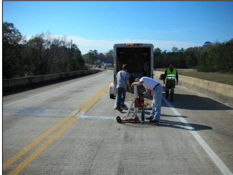
Figure 3-26: View of the bridge deck on SR 21 over CSXT Railroad at Tunnel Springs
