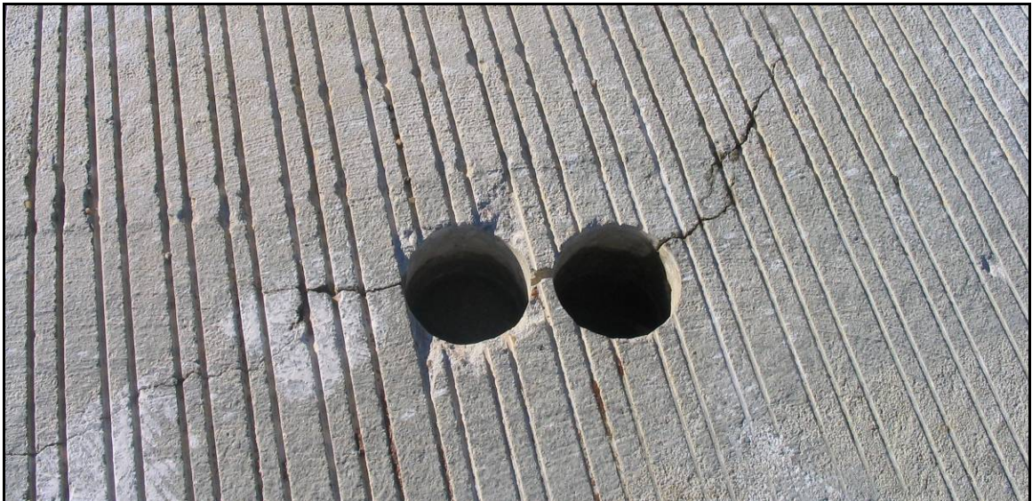
Figure 1-1: Core holes through cracks in the US 331 bridge deck
