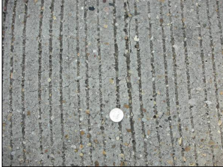
Figure 3-30: Picture of the surface cracking on the US 98 bridge deck
