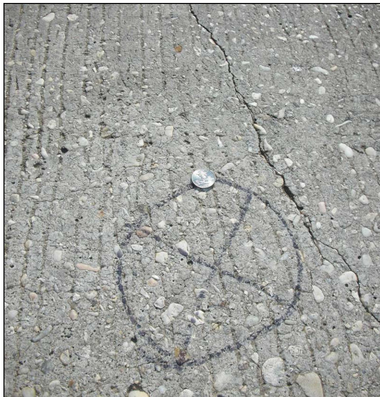
Figure 3-27: Picture of a wide surface crack on the SR 21 bridge deck at Tunnel Springs
