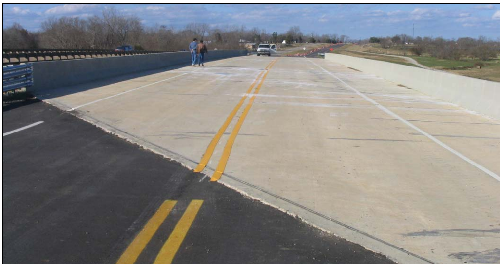
Figure 3-1: View of the northbound roadway bridge over the CSXT railroad on US 331
