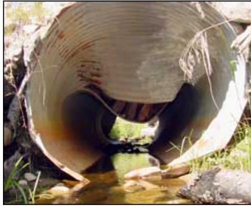
Figure 1. Example of collapsed culvert ( www.mnr.gov.on.ca/images )
