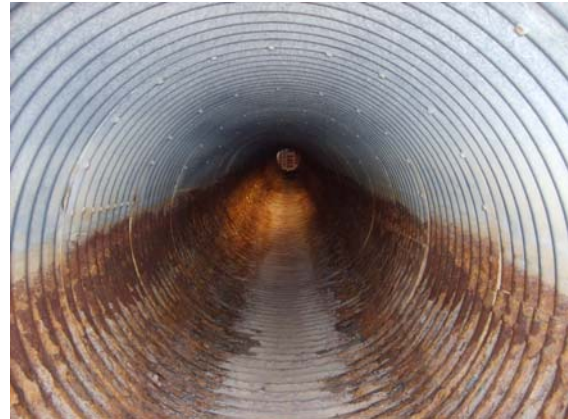
Figure 2B. Round culvert with rusted invert
