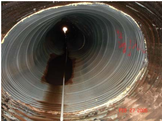
Figure 2A. Deformed culvert
