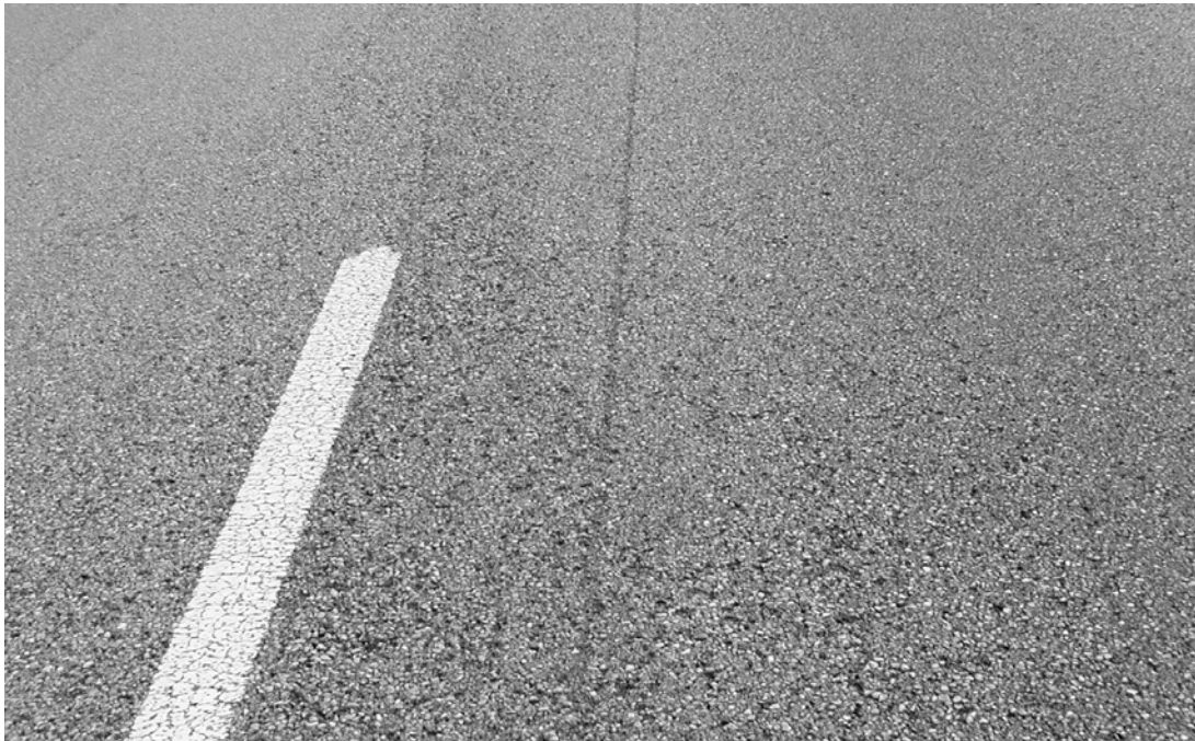
Figure 3.6 Photograph Showing Slight loss of Coarse Aggregate Particles in Section W10.
