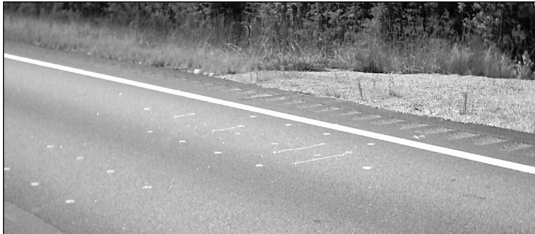
Figure 4.38 Transverse Cracking in the Wheelpath - Section N8.
