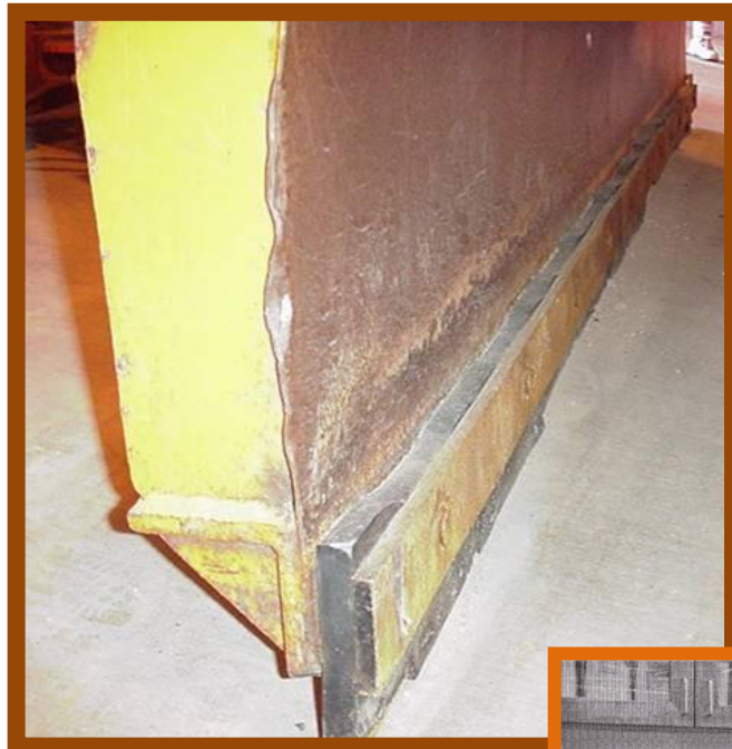
Corrosion on snow plow blade
