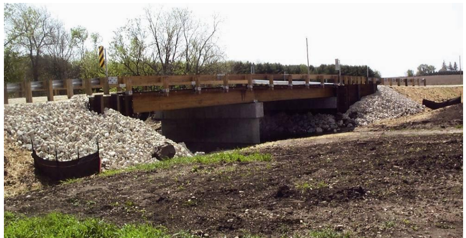
Demonstration timber bridge completed in spring 2009, Delaware County, Iowa, features an innovative deck treatment system
