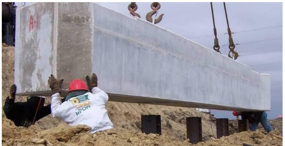
Boone County bridge substructure (West abutment) being placed Photos: Dr. Terry Wipf, Iowa State University/BEC
