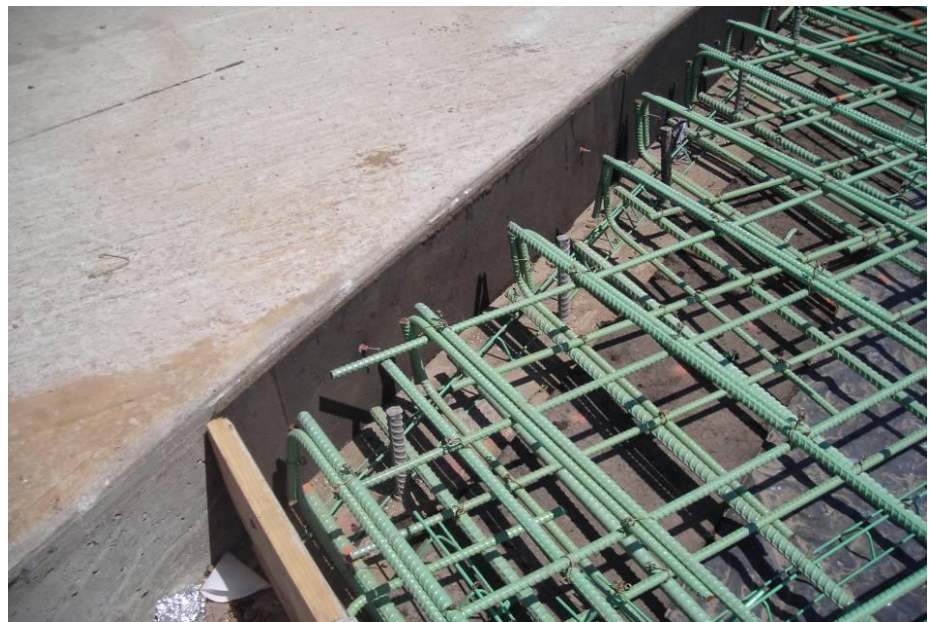
Installation of an improved bridge-to-pavement connection detail Photo: Dr. Brent Phares, Iowa State University/CCEE
