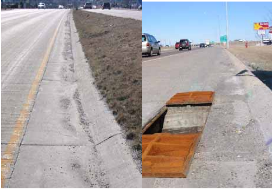
Figure 5. Street-dirt at the swept sections median; the un-sweep east bound curb near the water-quality manhole.
