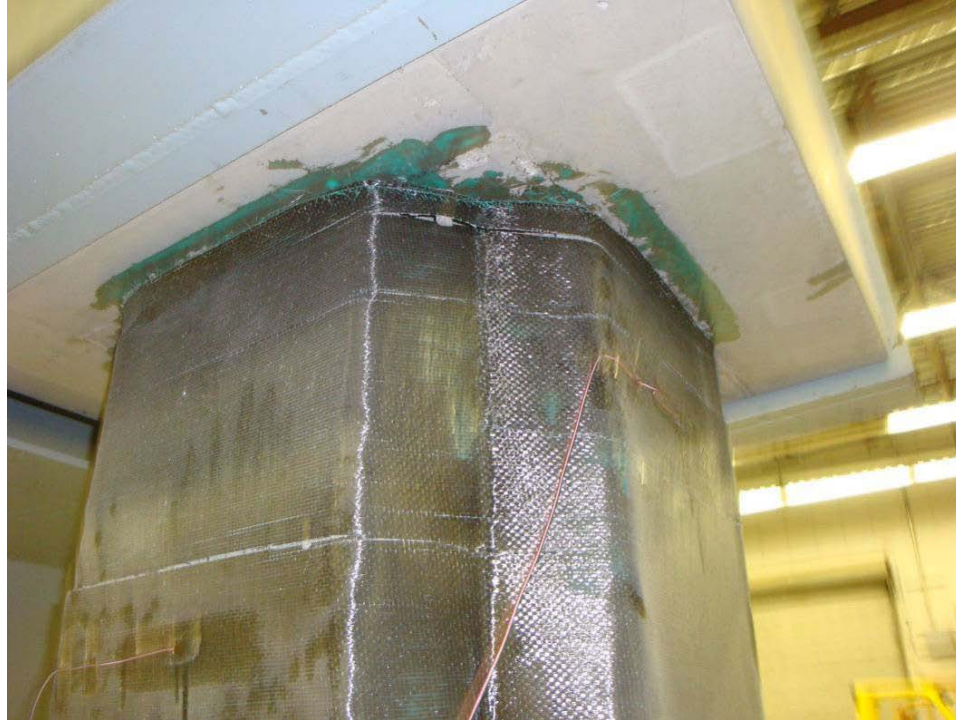
Figure 28 – Column 2 Pullout of FRP Jacket from Reentrant Corners
