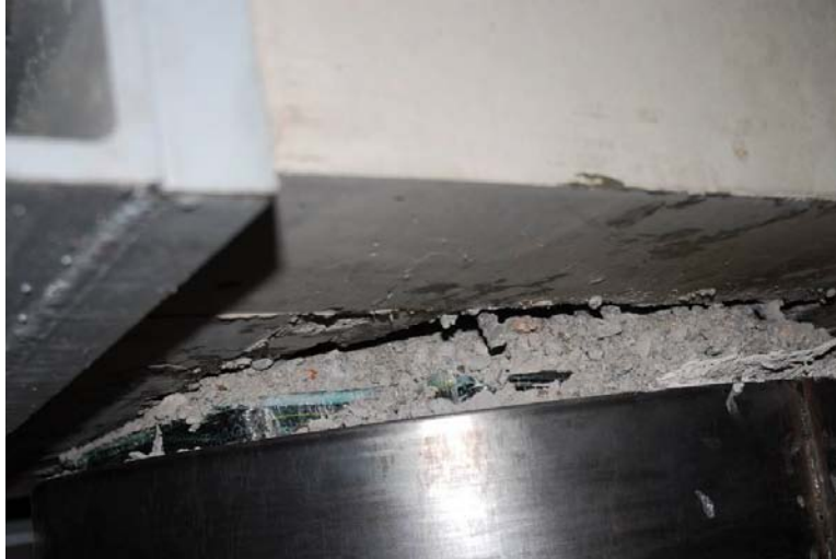
Figure 43 – Column 4 Longitudinal Rebar Fracture
