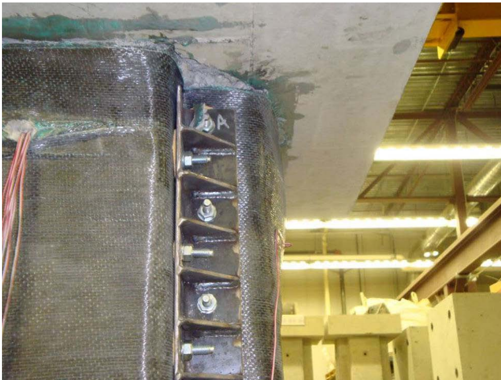
Figure 36 – Column 3 Bulging of FRP Jacket at the Top of the Column
