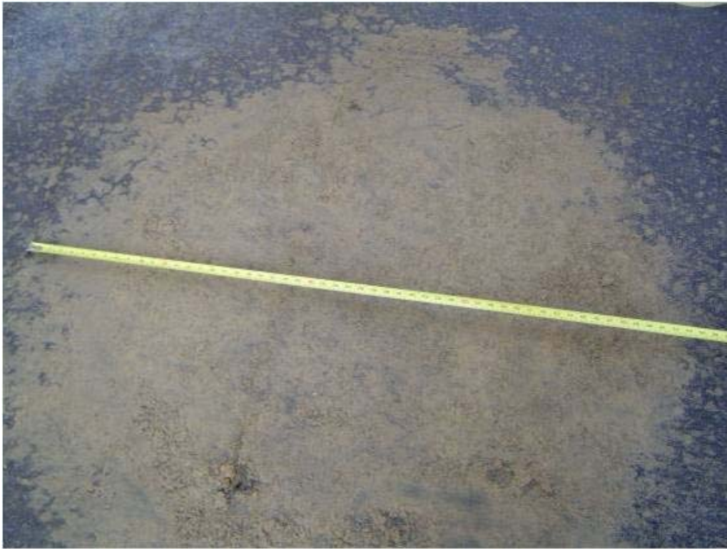
Figure 92. Fabric Stained by Pumped Subgrade Fines - Post 19" ABC with Geotextile A (6) Test
