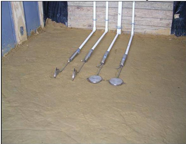
Figure 51. Installed Earth Pressure Cells (EPCs)
