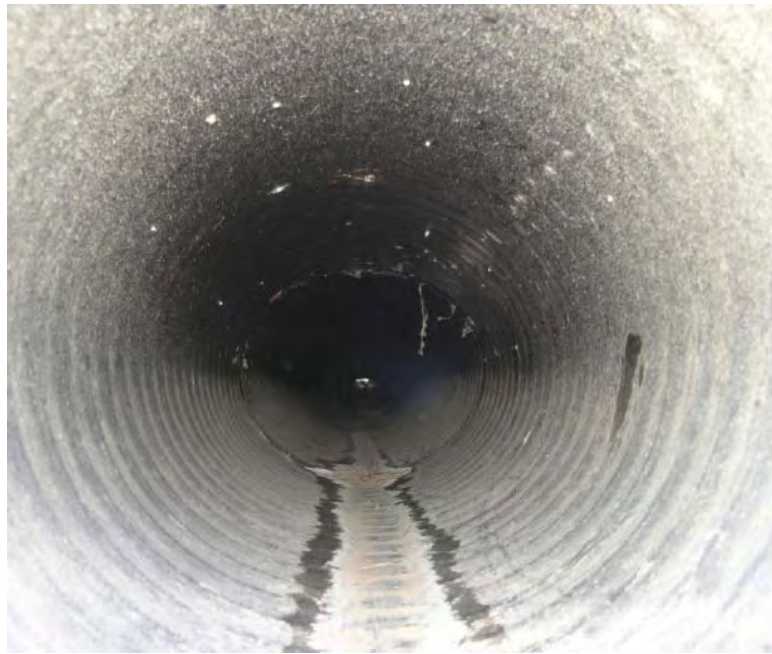
Figure 9. Photo through culvert showing sag.
