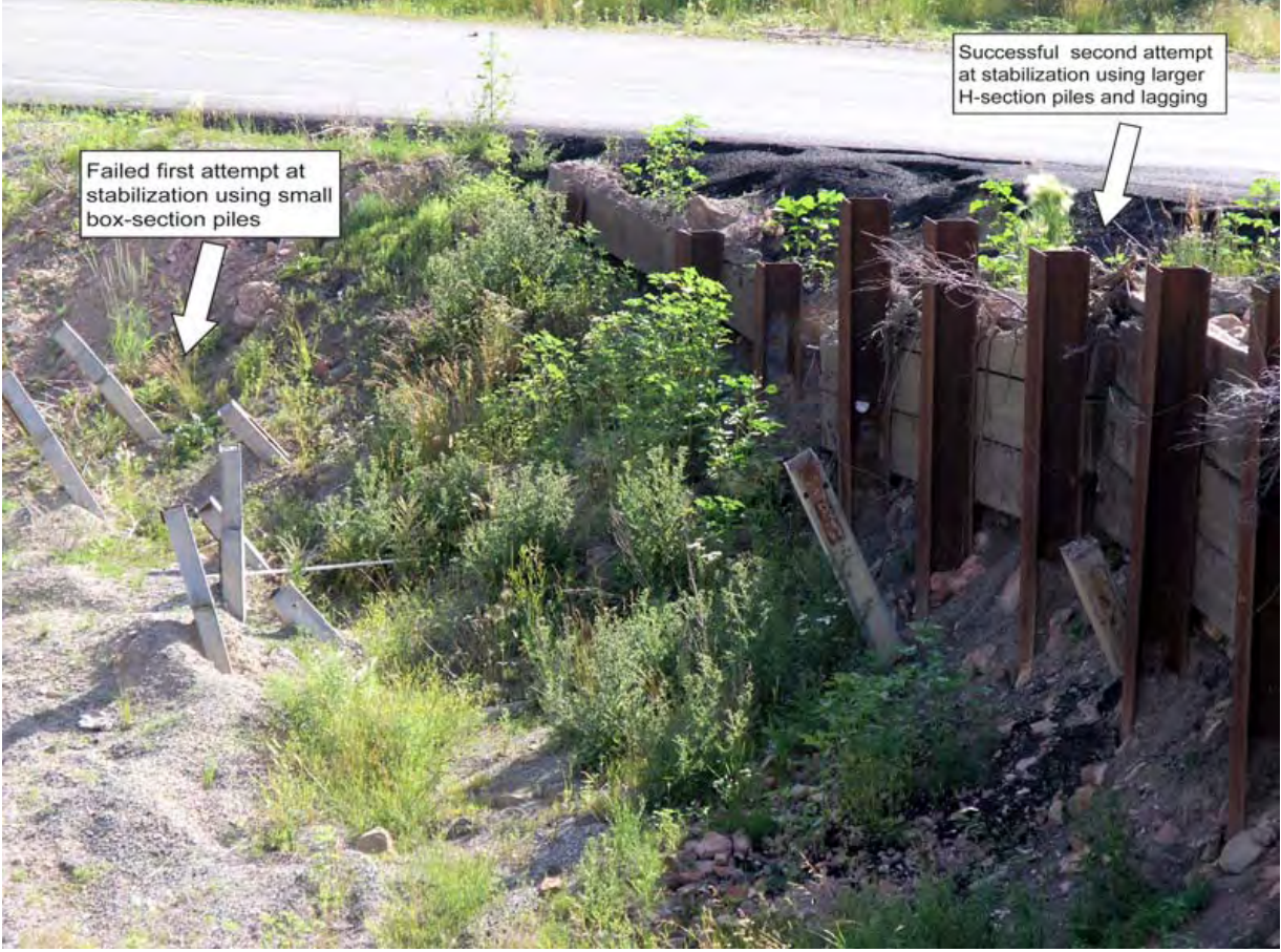
Figure 14. Stabilized site at Douglas Pass, showing failed first attempt.
