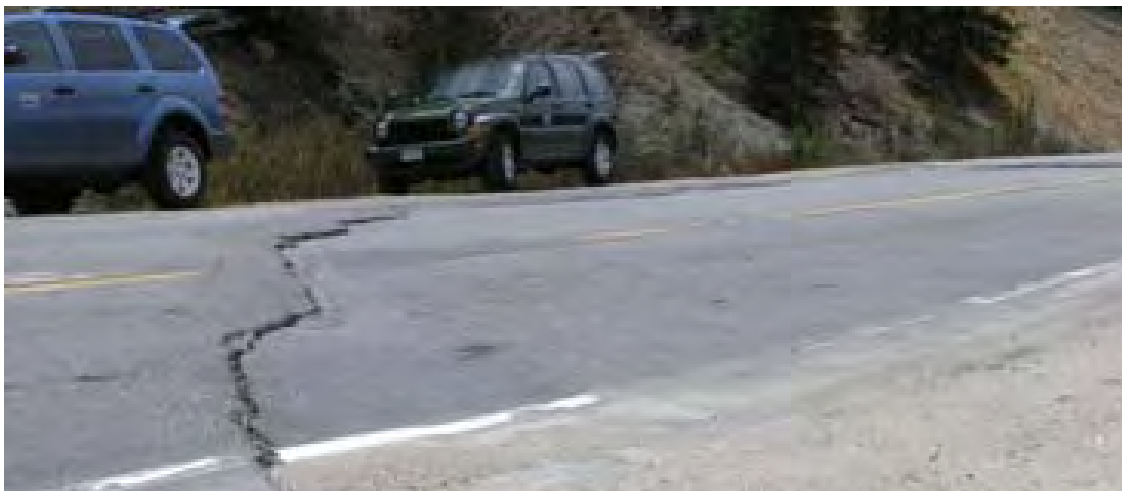
Figure 11. Pavement distress at Hoosier Pass.
