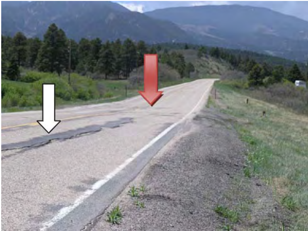
Figure 8. Pavement distress at Rye (2009).
