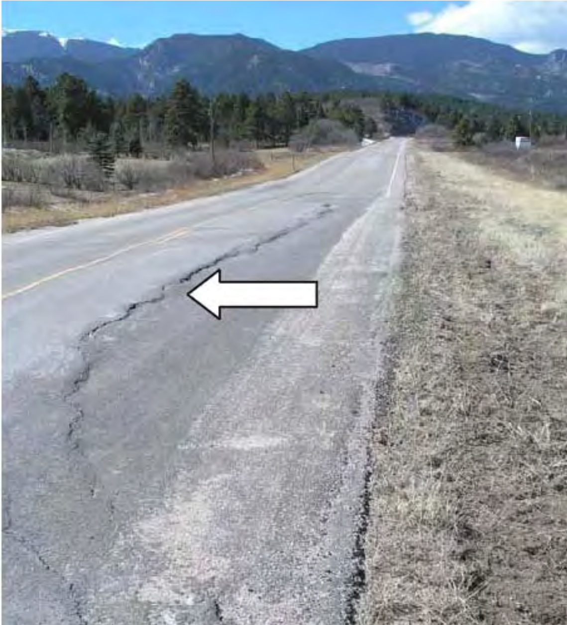
Figure 7. Pavement distress at Rye (2006).
