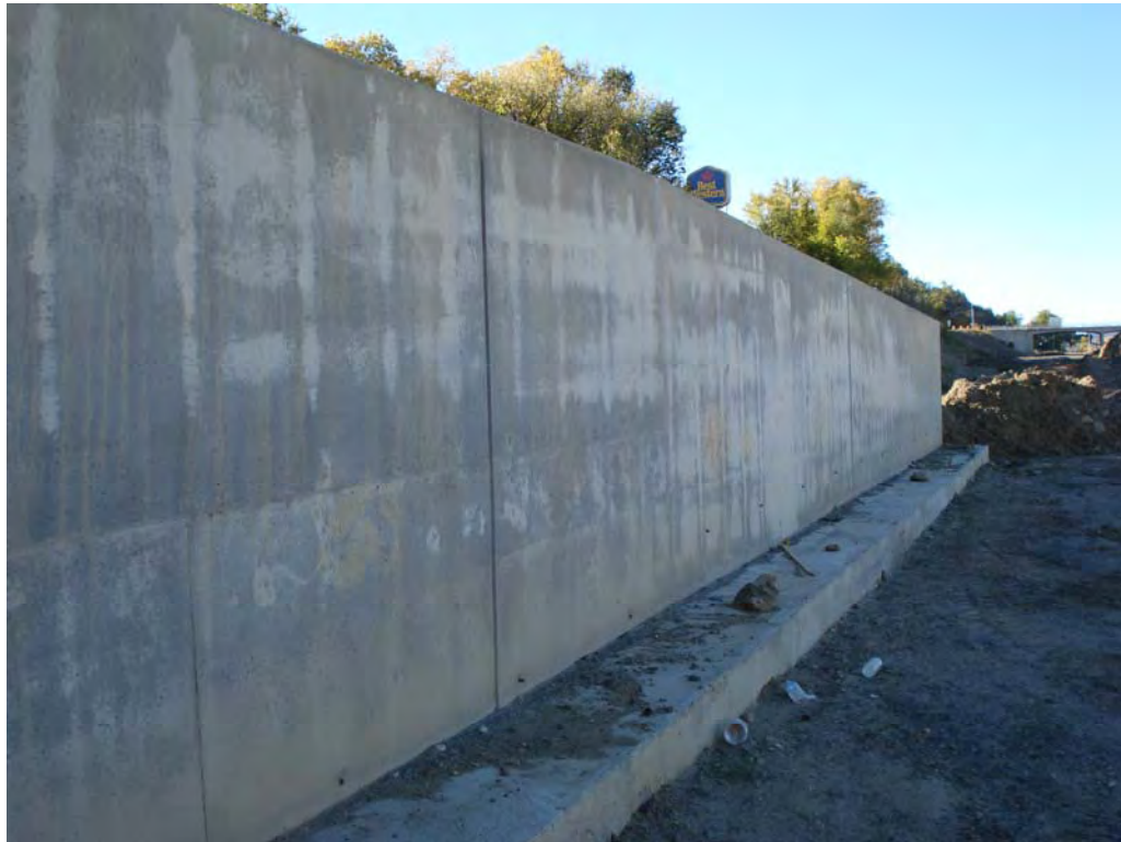
Figure 11: Discolorations on Retaining Wall
