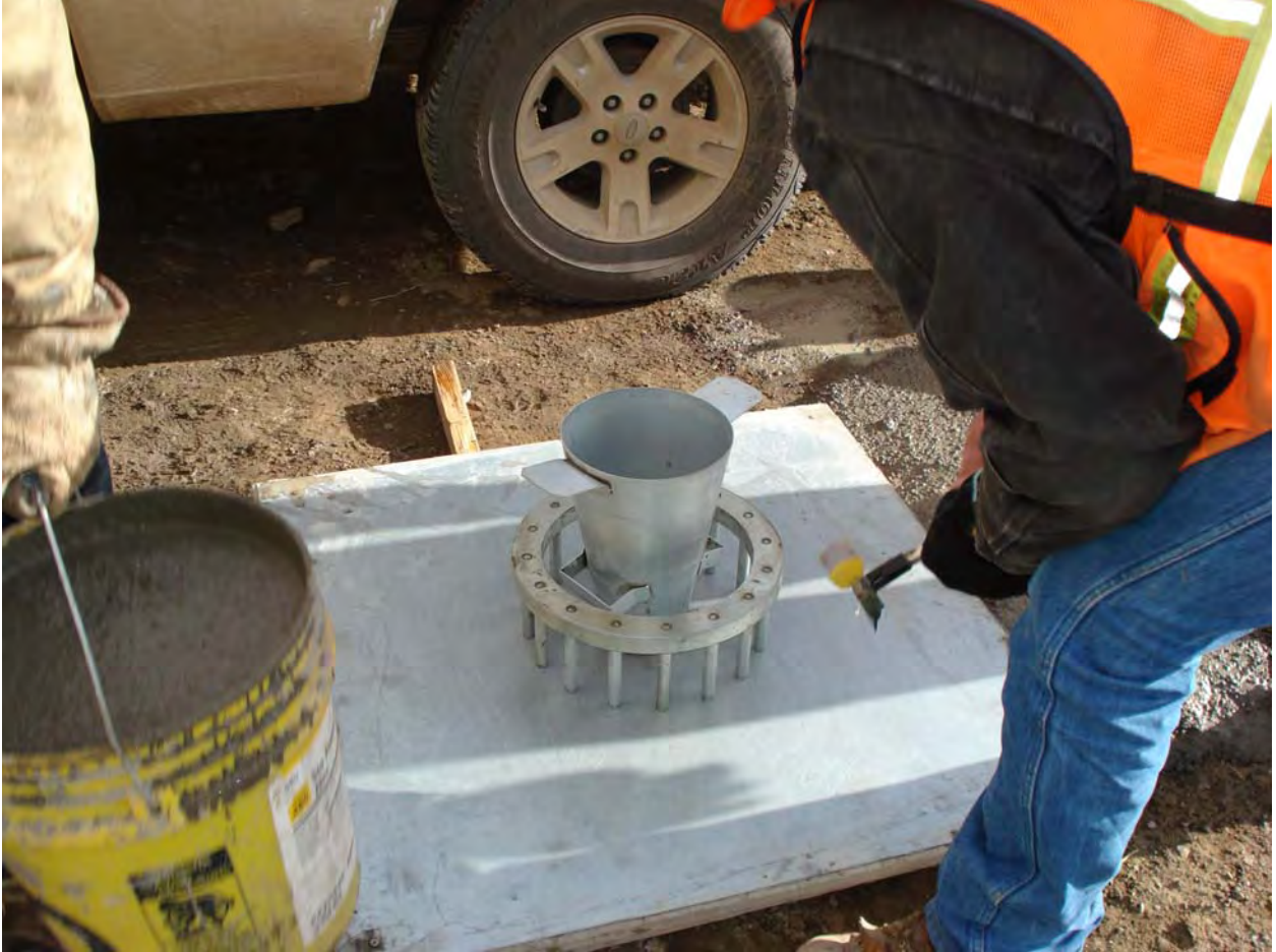
Figure 1: Abrams Cone and J-Ring for Slump Flow Test
