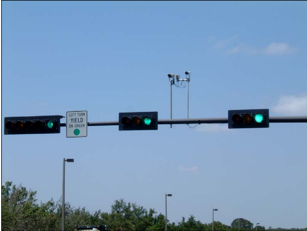
Figure 27. Mounting Arrangement of the Test Cameras.
