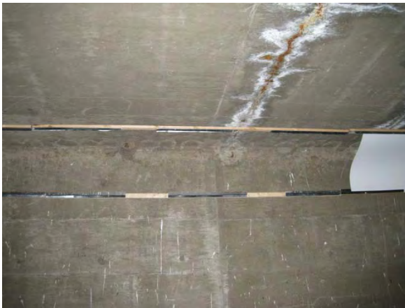
Figure 27. Swallow nests on the south side of CBC 4 in the space where white plastic panels had fallen down.
