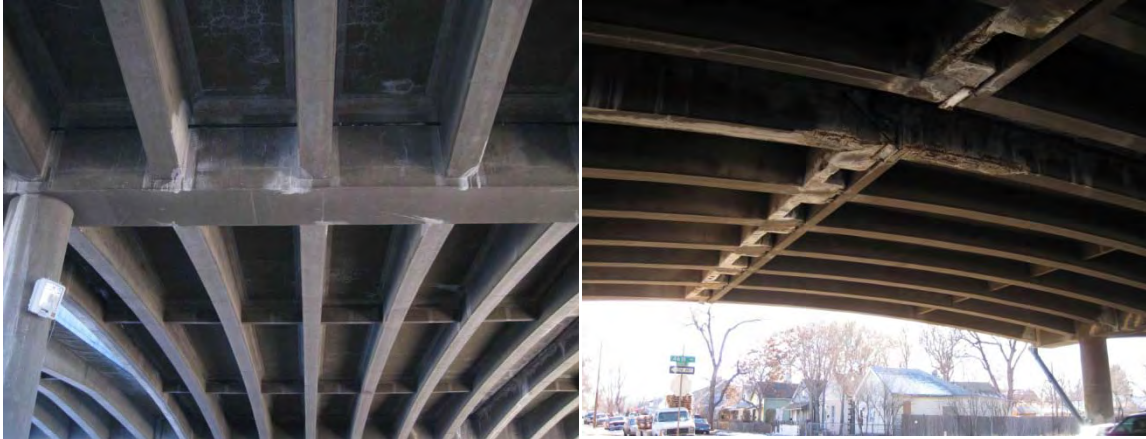
Figures 8 and 9. The underside of I-70 showing an old poured in place concrete structure that effectively deters pigeon nesting/roosting, but deteriorates over time.
