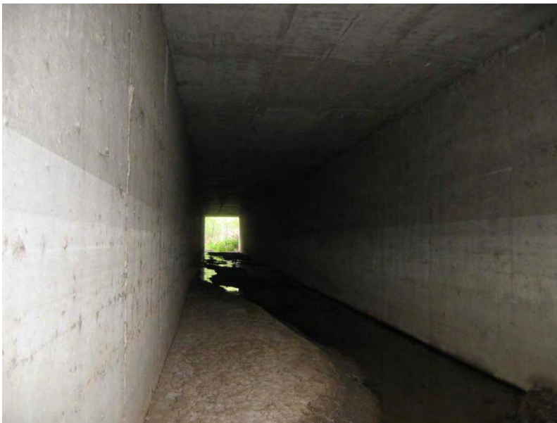
Figure 13. Looking west in CBC 3 used as a control; this is the northernmost of the three parallel CBCs.
