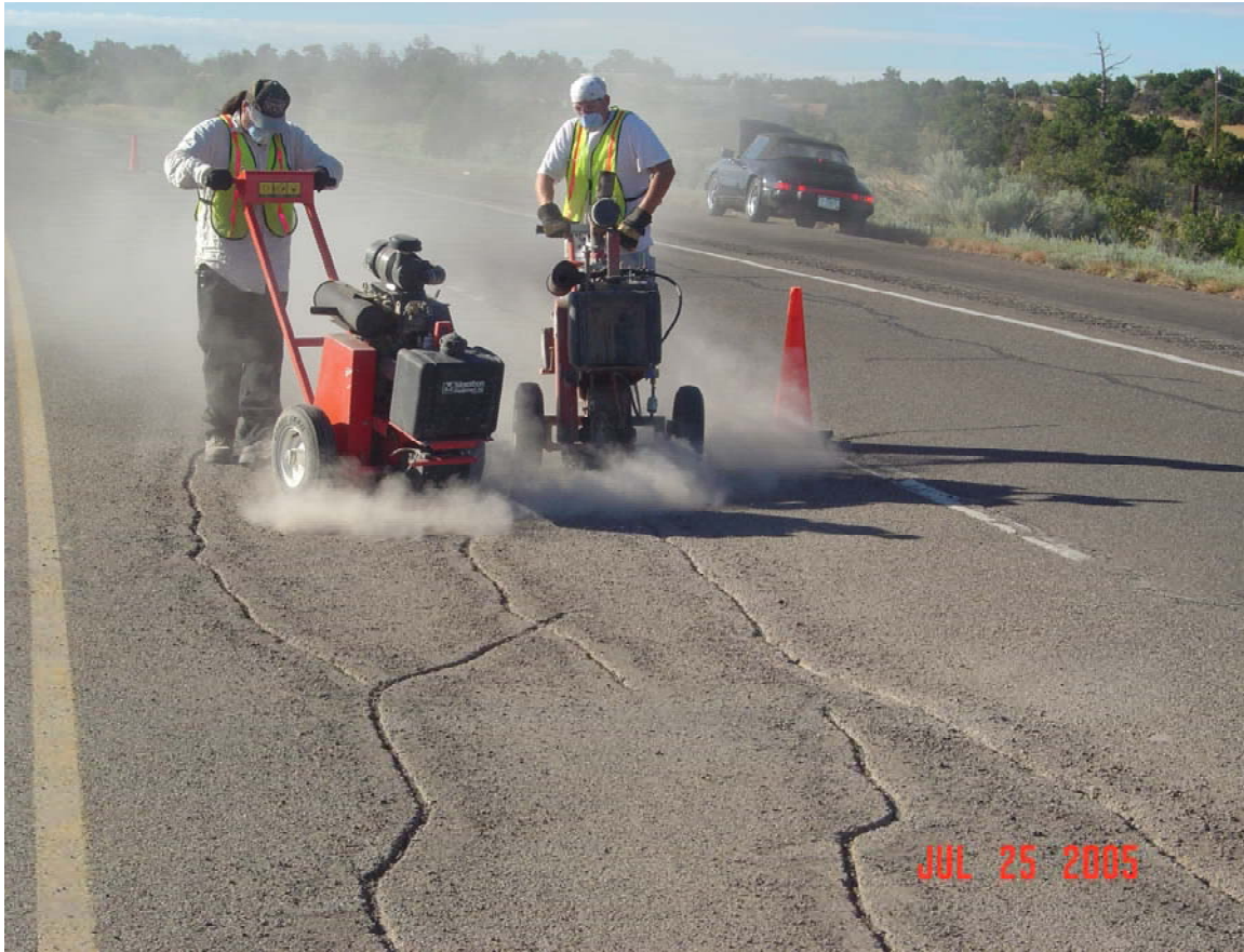
Figure A1 – Routing Cracks Prior to Crack Sealer Installation on I-25, NM
