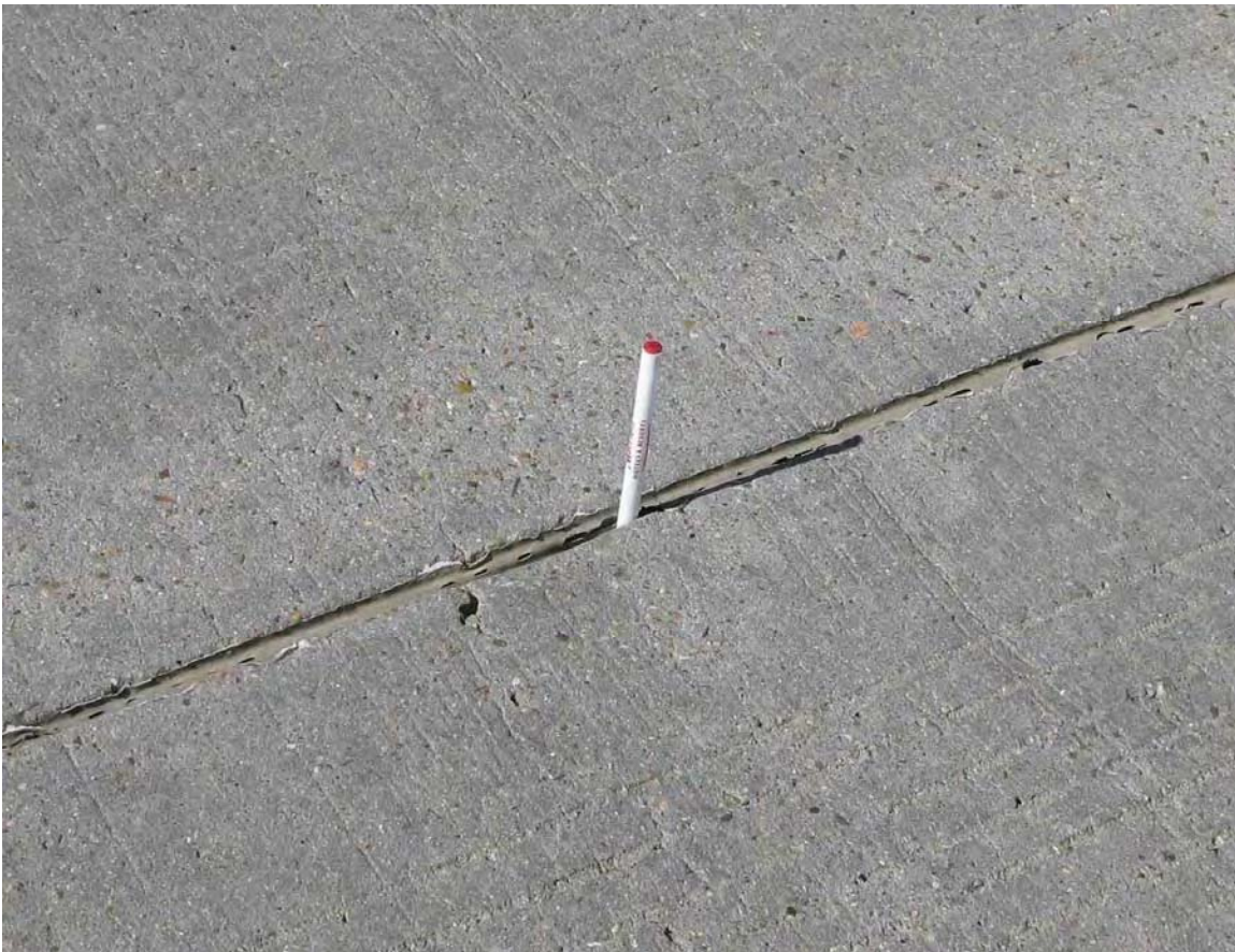
Figure 120. Sealant Failure on US 287, Campo
