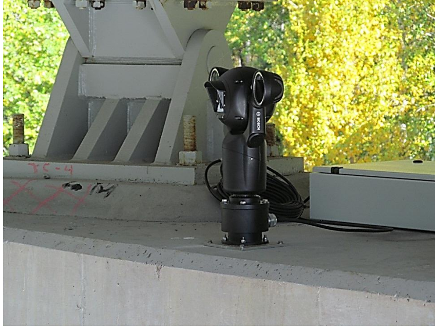
Figure 10. Camera and Camera Control Panel
