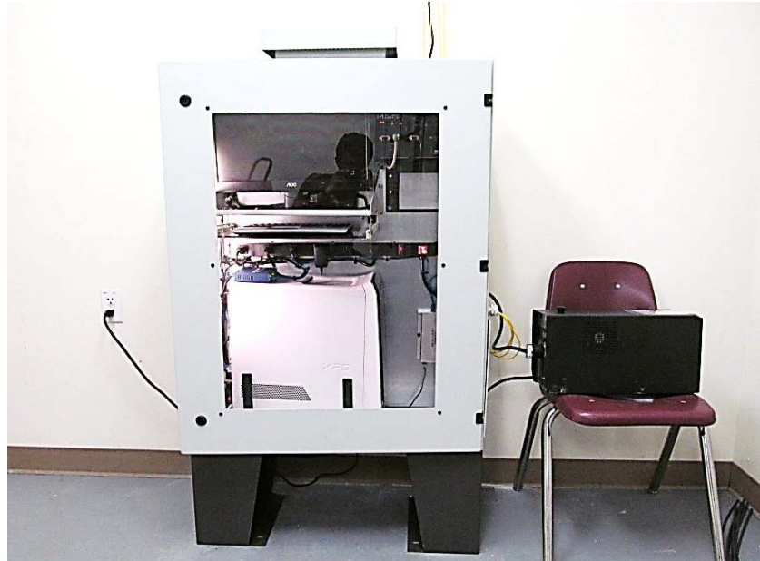
Figure 9. Control Panel at the Princess Hotel
