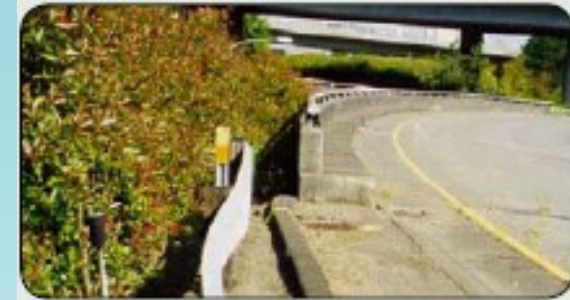
Before: Outdated guardrail at the SR 7/SR 705 interchange with I-5 in Tacoma.
