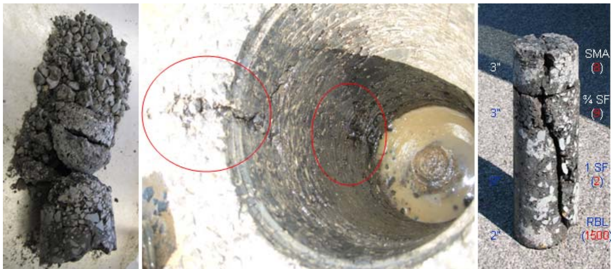
Figure 5-3. Coring along the Longitudinal Crack on IH 35 (Gilbert Job).
