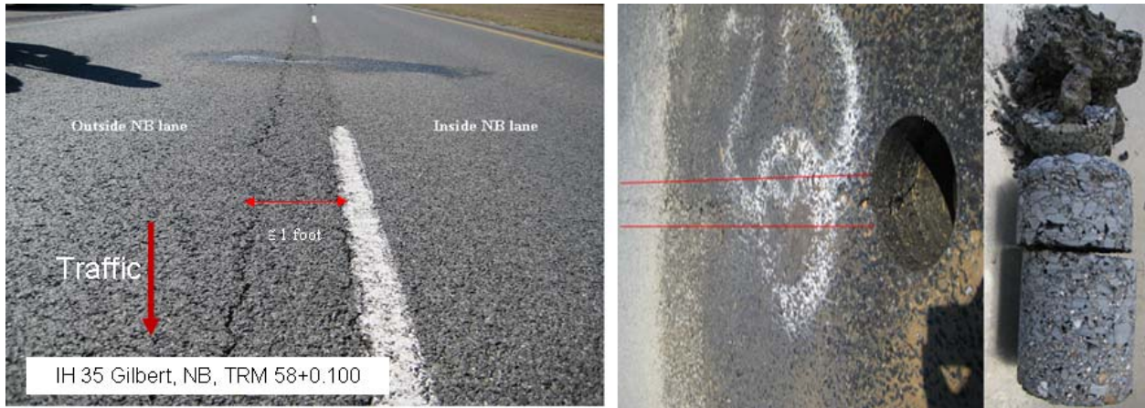
Figure 5-2. Longitudinal Cracking on IH 35 (Gilbert Job).
