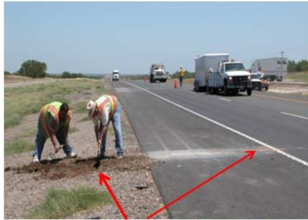
MDD connector cables being buried for subsequent measurements
