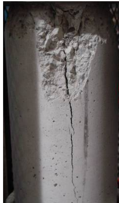
(b) Failure mode
