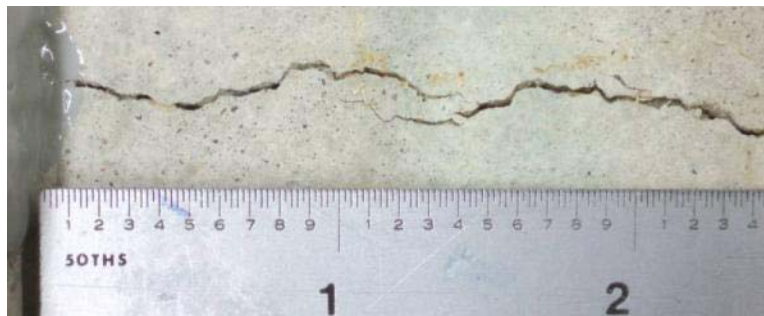
Figure 6.44 Cracking along the surface of the specimens with uncoated reinforcement.
