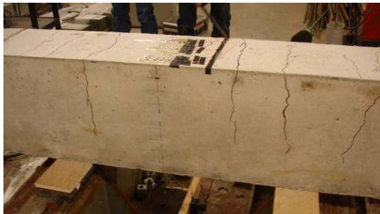
(b) Initial cracks
