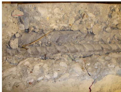
Figure 5.13 Enamel coating remained on steel rebar.
