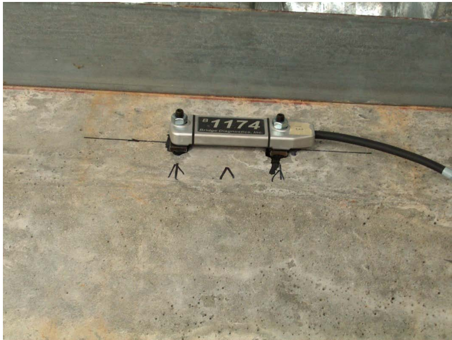
Figure 172 Gauge located at the top flange of the Girder 4
