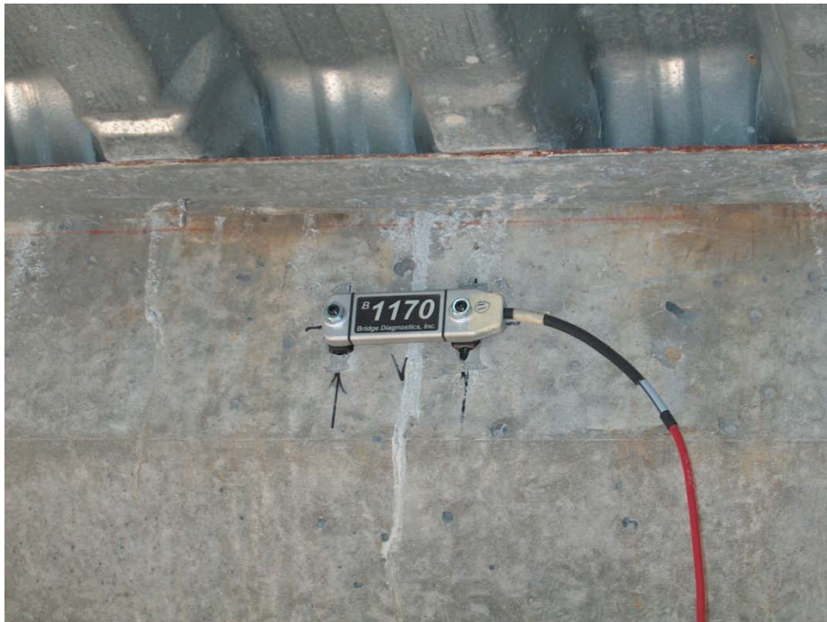
Figure 166 Gauge located at the top flange of the Girder 3
