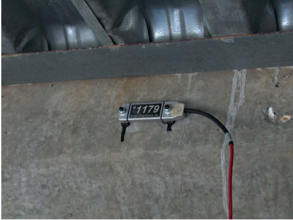
Figure 183 Gauge located at the top flange of the Girder 6
