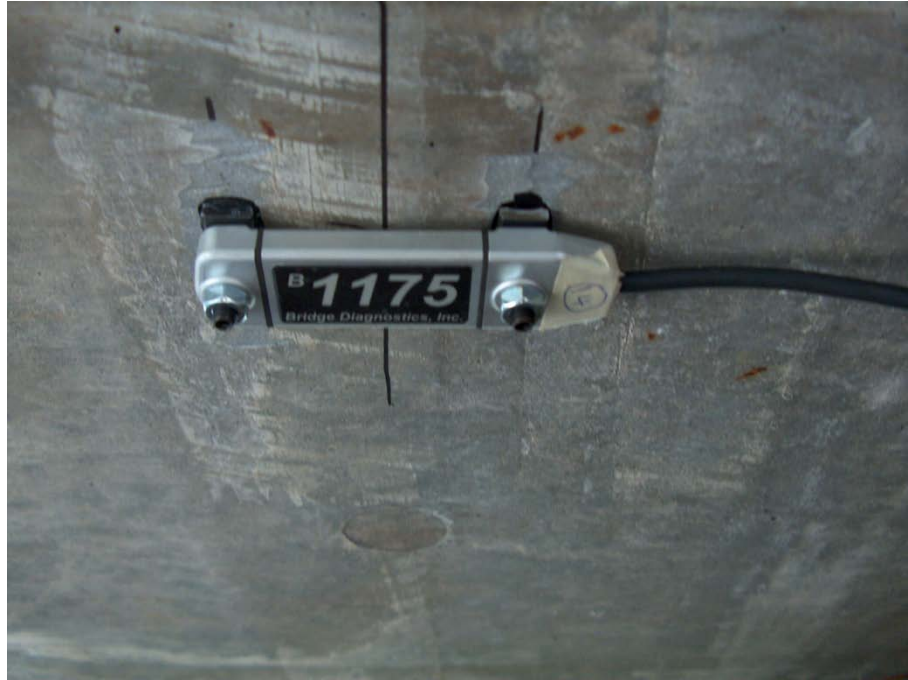
Figure 175 Gauge located at the bottom of the Girder 4
