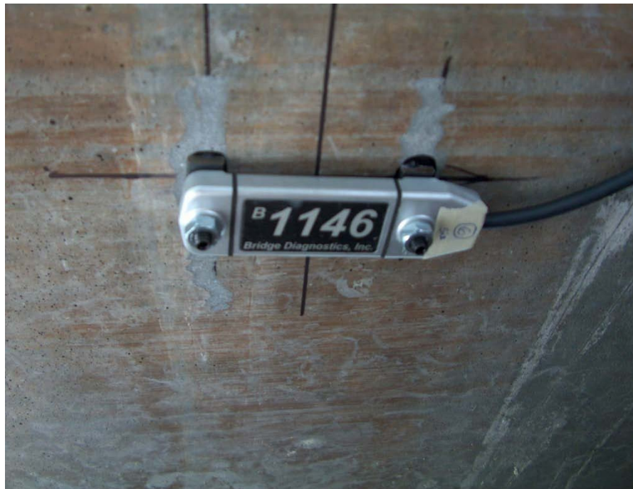
Figure 158 Gauge located at the bottom of the Girder 2
