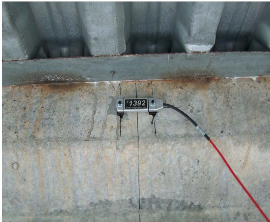
Figure 162 Gauge located at the top flange of the Girder 2
