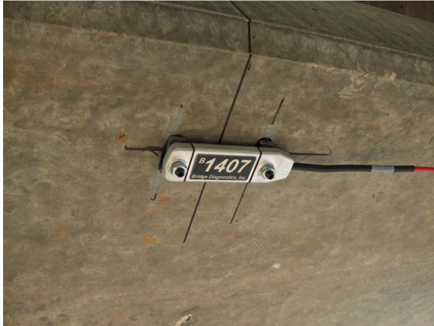
Figure 141 Gauge located at the bottom of the Girder 1
