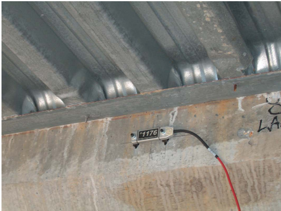
Figure 178 Gauge located at the top flange of the Girder 1
