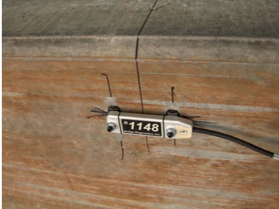
Figure 163 Gauge located at the bottom of the Girder 2
