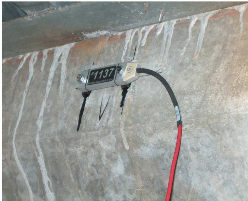
Figure 144 Gauge located at the top flange of the girder
