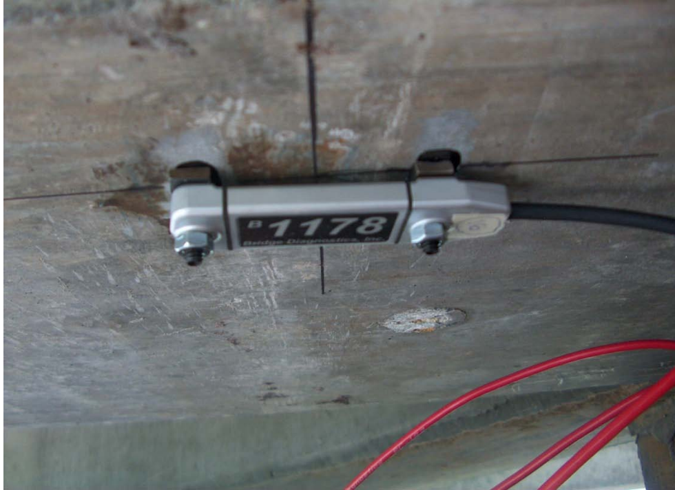
Figure 181 Gauge located at the bottom of the Girder 5
