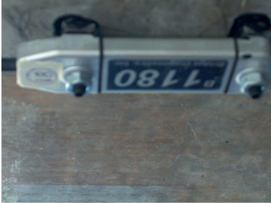
Figure 185 Gauge located at the bottom of the Girder 6
