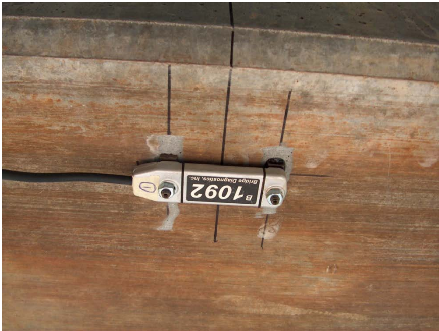
Figure 152 Gauge located at the bottom of the Girder 1
