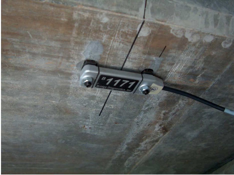
Figure 169 Gauge located at the bottom of the Girder 3
