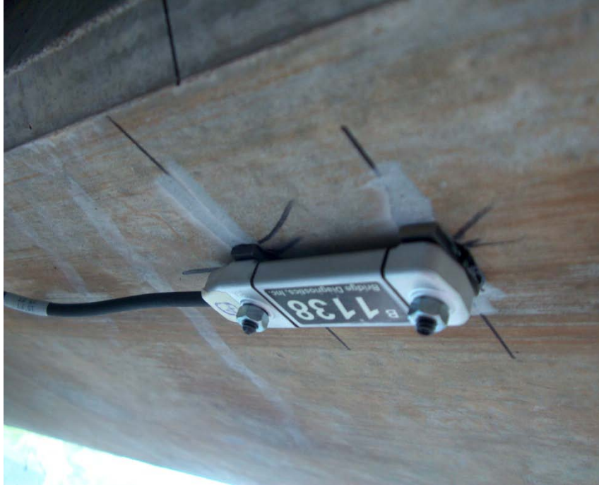
Figure 147 Gauge located at the bottom of the Girder 1
