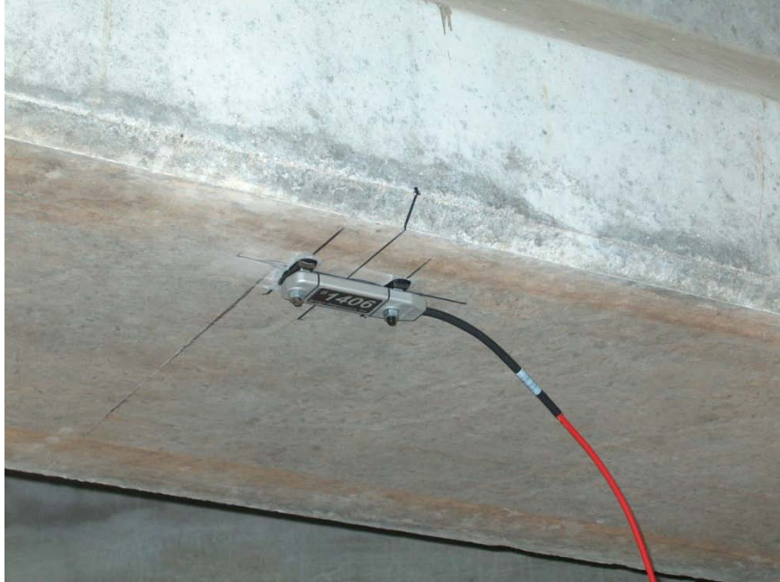
Figure 155 Gauge located at the bottom of the Girder 2
