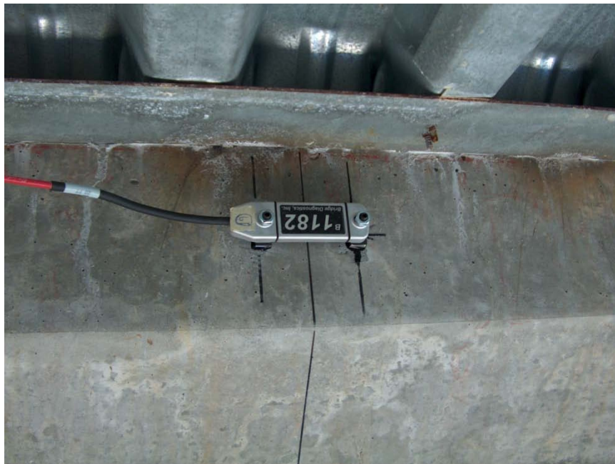
Figure 150 Gauge located at the top flange of the Girder 1
