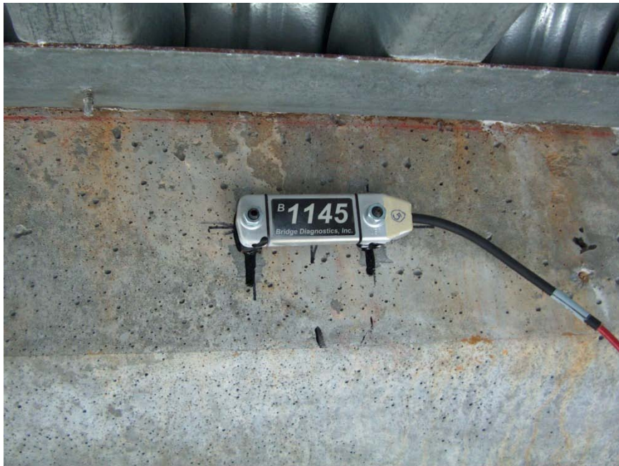
Figure 156 Gauge located at the top flange of the Girder 2
