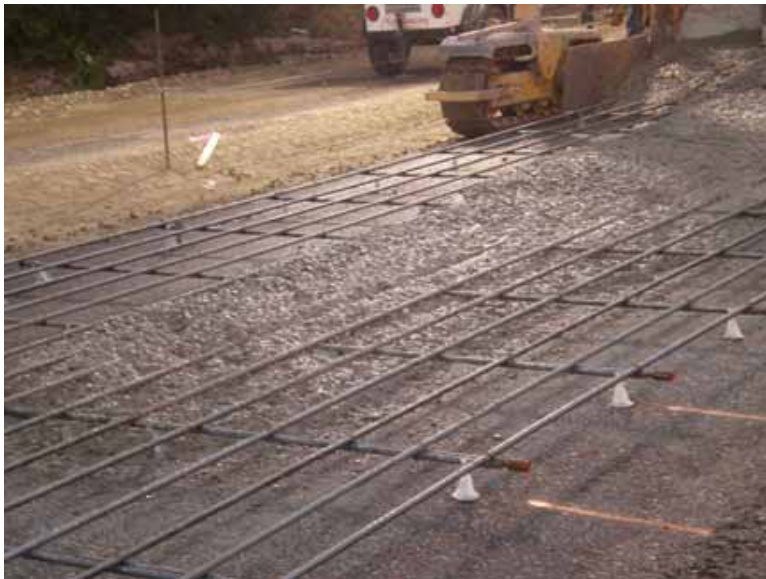
Figure B8. Concrete mixture with too much water
