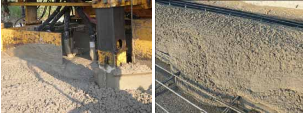
Figure B13. Segregation due to high water content
