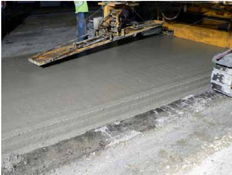
Figure B12. Concrete straight from the paver before workers began with final finishing
