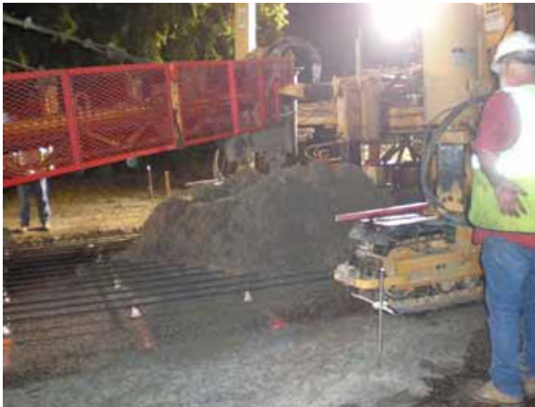
Figure B4. Extremely low slump on one of the first truck loads
