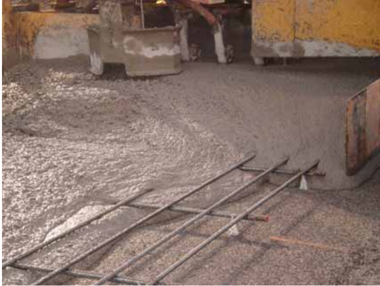
Figure B9. Poor concrete with visible segregation due to high water content
