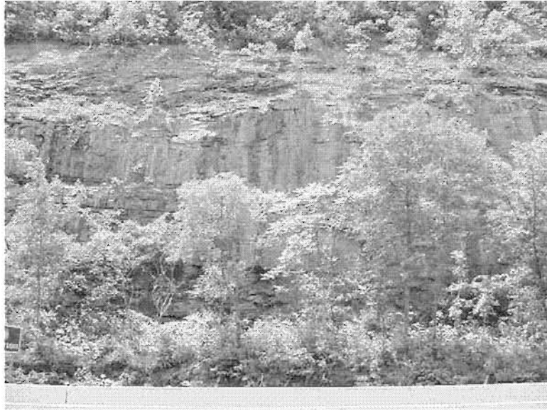
Figure F-15: JEF-7-28a, high hazard potential (117)
