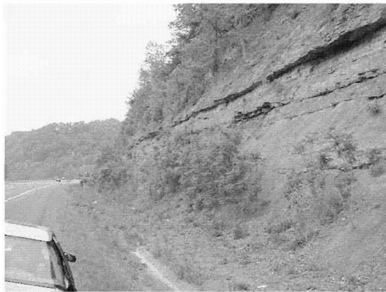
Figure F-22: JEF-7-22.6, high hazard potential (106)
