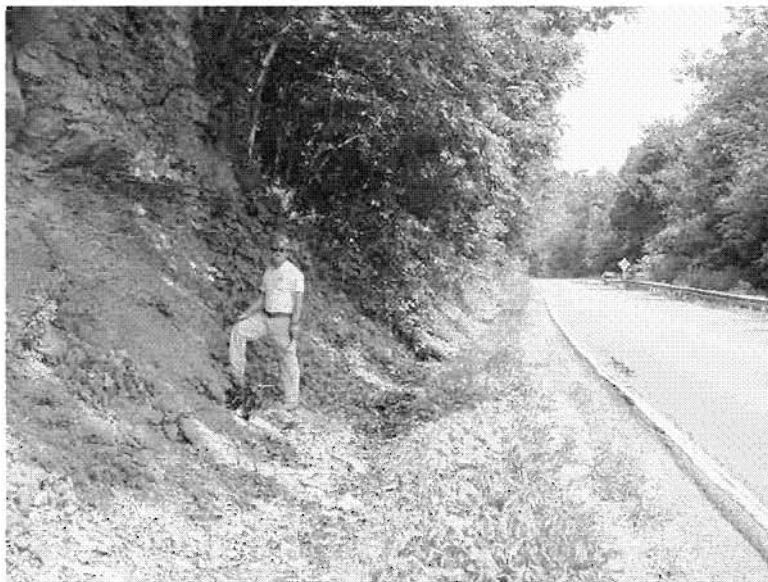
Figure F-66: ATH-13-13.7, moderate hazard potential (71)
