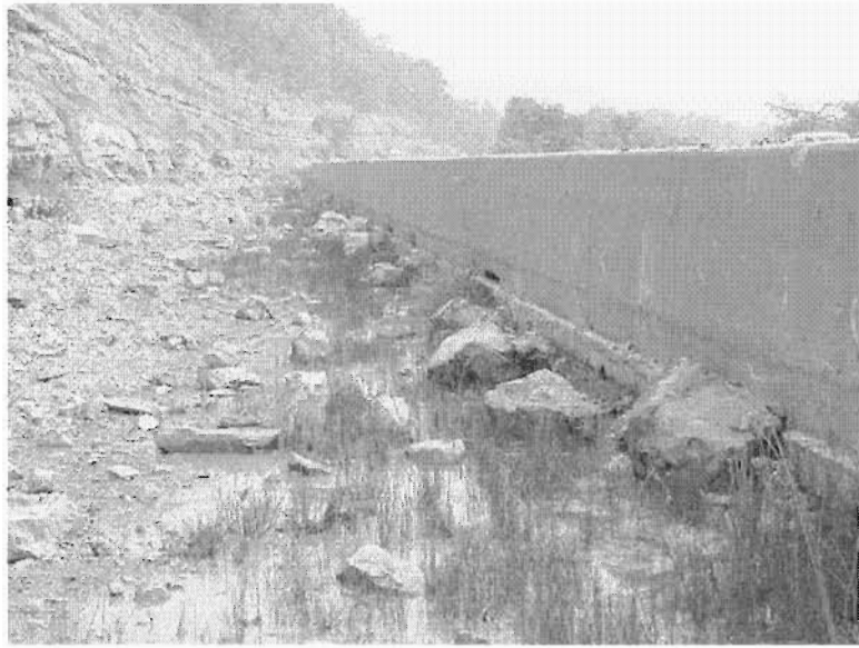
Figure F-27: BEL-7-11, moderate hazard potential (98)
