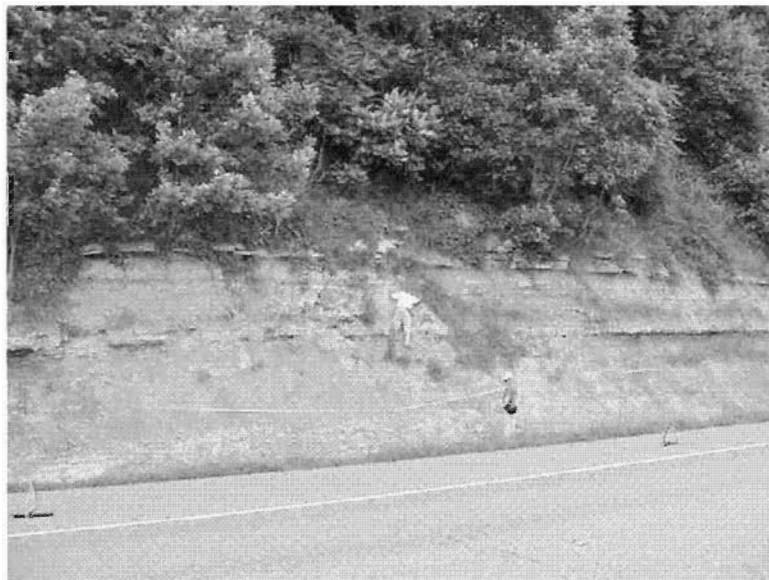
Figure F-86: BEL-7-5.9, moderate hazard potential (56)
