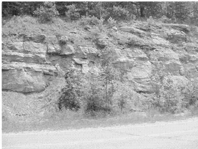
Figure F-84: PER-13-5.1, moderate hazard potential (57)
