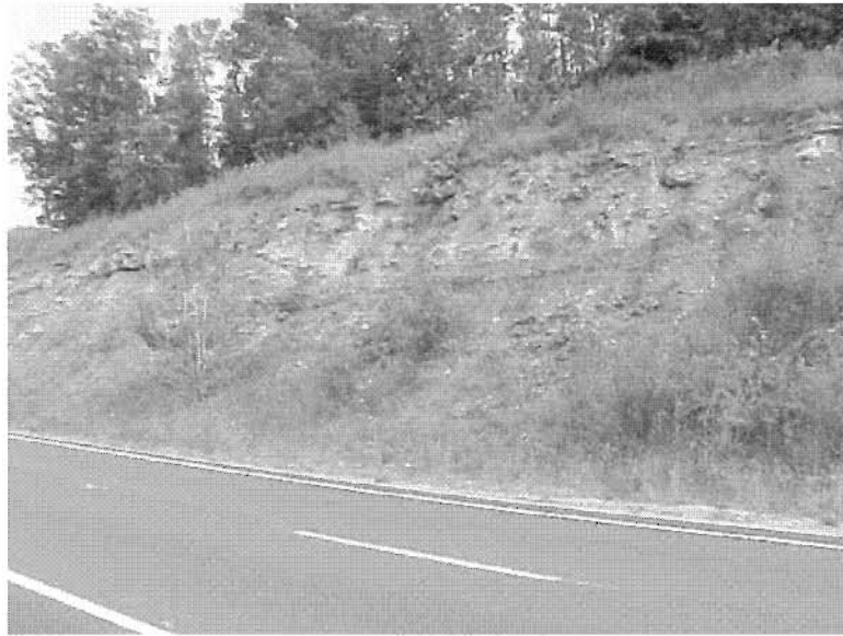
Figure F-77: PER-155-1.83, moderate hazard potential (61)
