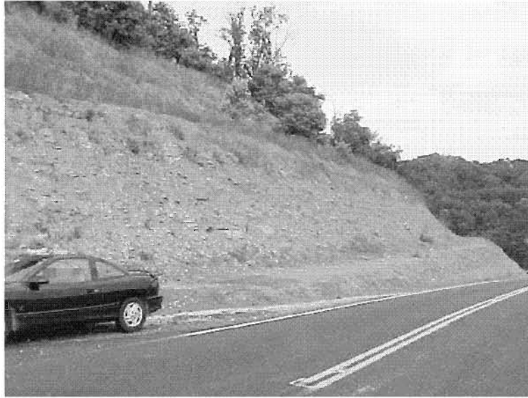
Figure F-43: COS-715-6.5, moderate hazard potential (90)
