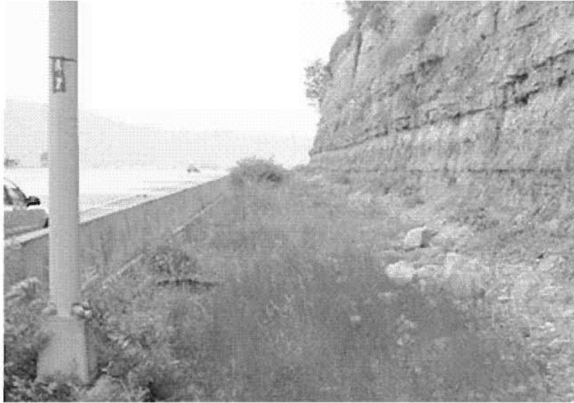
Figure F-73: BEL-7-14, moderate hazard potential (64)
