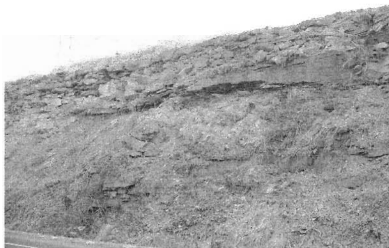
Figure F-28: WAY-21-2.36, moderate hazard potential (98)
