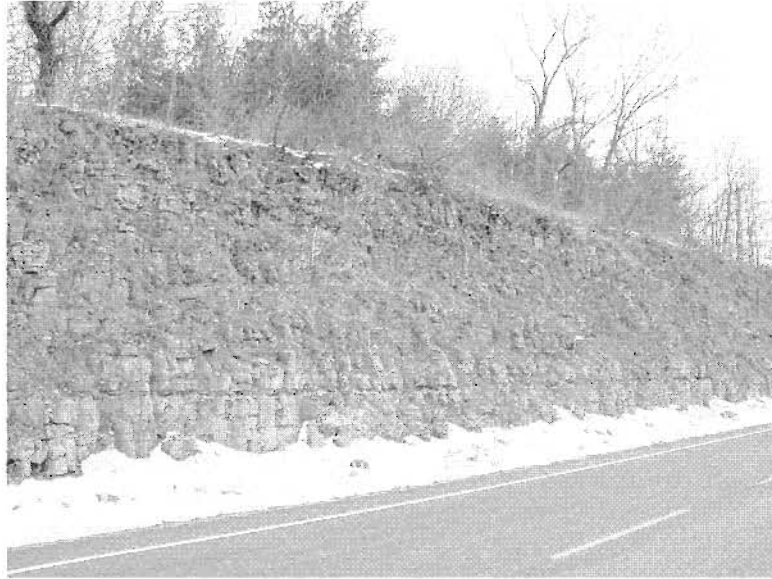
Figure F-49: LOG-292-2.6, moderate hazard potential (84)
