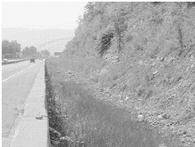
Figure F-70: BEL-7-9, moderate hazard potential (66)
