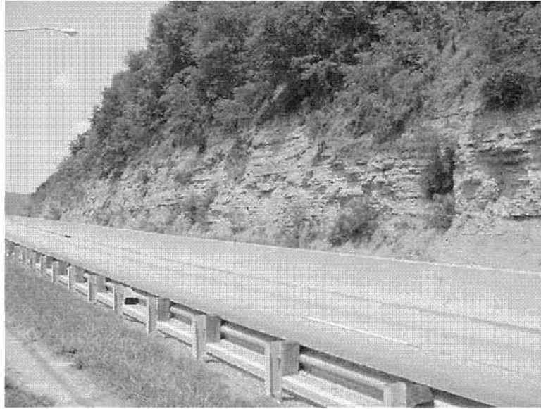
Figure F-65: SCI-52-25.5B, moderate hazard potential (72)
