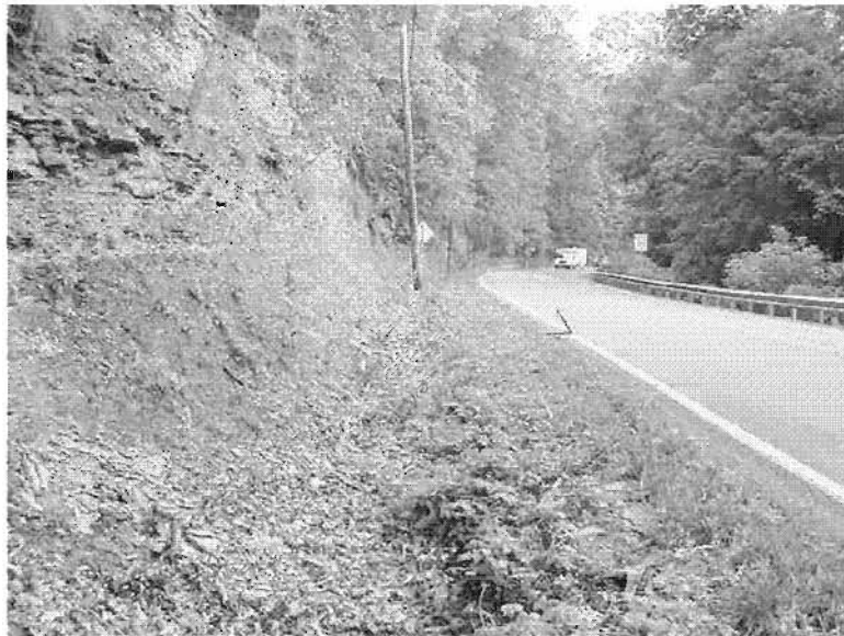
Figure F-44: ATH-13-9.2, moderate hazard potential (87)
