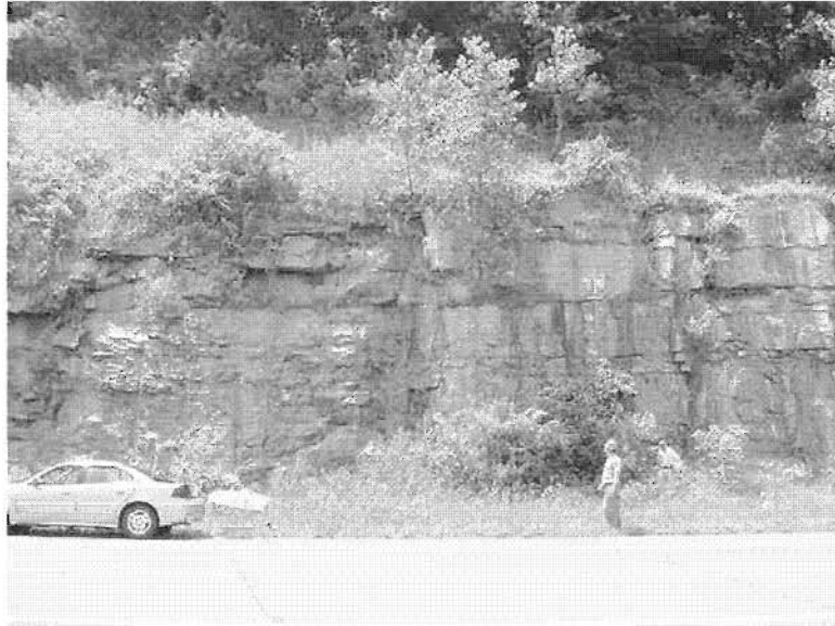
Figure F-61: BEL-7-18.6, moderate hazard potential (73)
