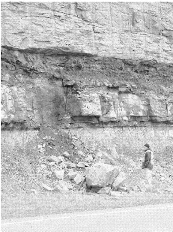
Figure F-42: BEL-149-1.8, moderate hazard potential (90)
