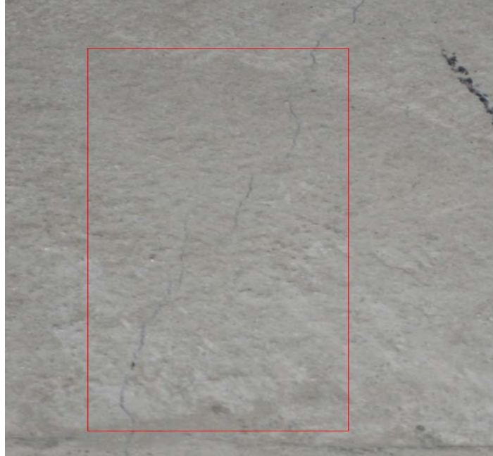
Figure 4.27 Crack in the middle of the slab caused by the restraints
