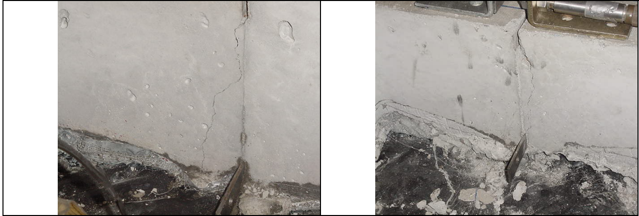
Figure 4.30 Close-up of induced crack for slab 4. Left: North Side; Right: South Side
