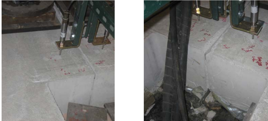
Figure 4.18 Close-up of induced crack. Left: North Side of Slab; Right: South Side of Slab
