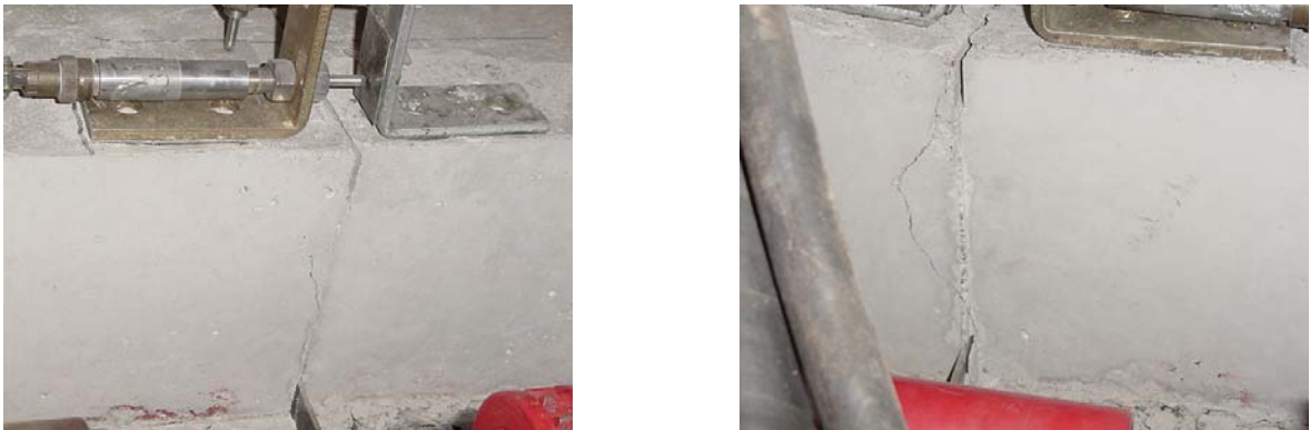
Figure 4.36 Slab 5 - Left: North Side of Crack, Right: South Side of Crack
