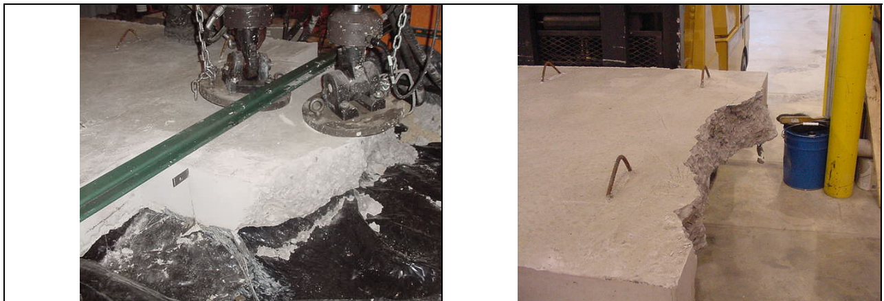
Figure4.35. Photo of Slab 3 Crack
