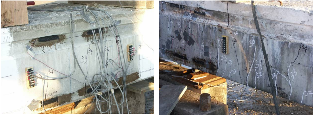
Photo 3-12. Flexural cracking at mid-span
