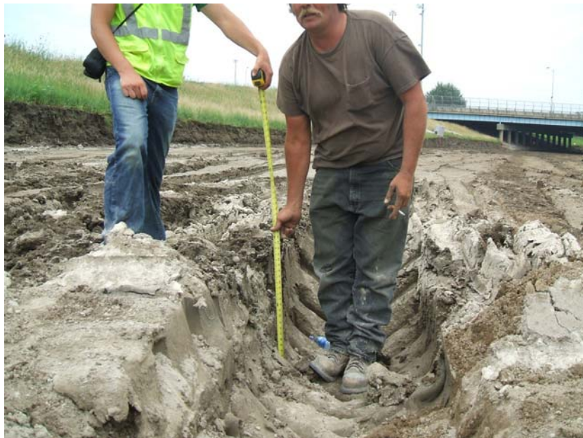
Figure 11: Ruts Caused by the Spreader Truck
