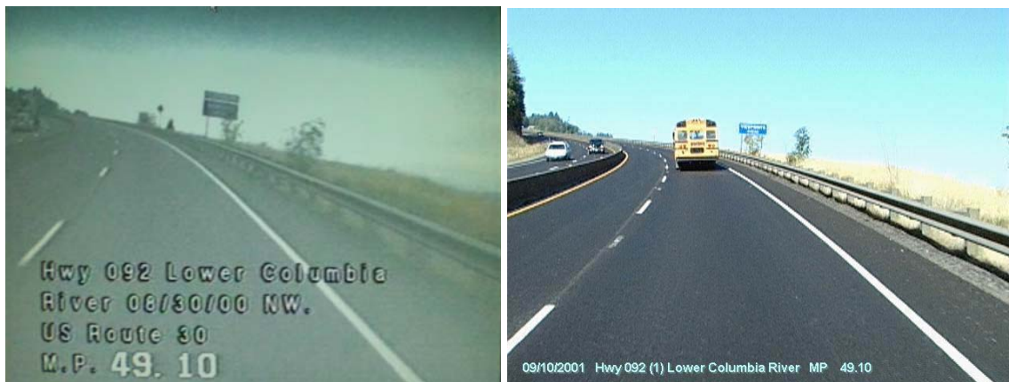
Figure 5.8: Conditions in 2000 (before) and 2006 (after) showing guardrail and pavement markings at MP 49.10
