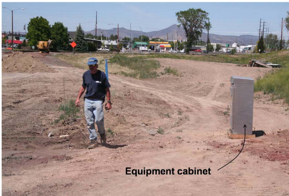
Figure 3.10: Equipment cabinet at the Redmond test site.
