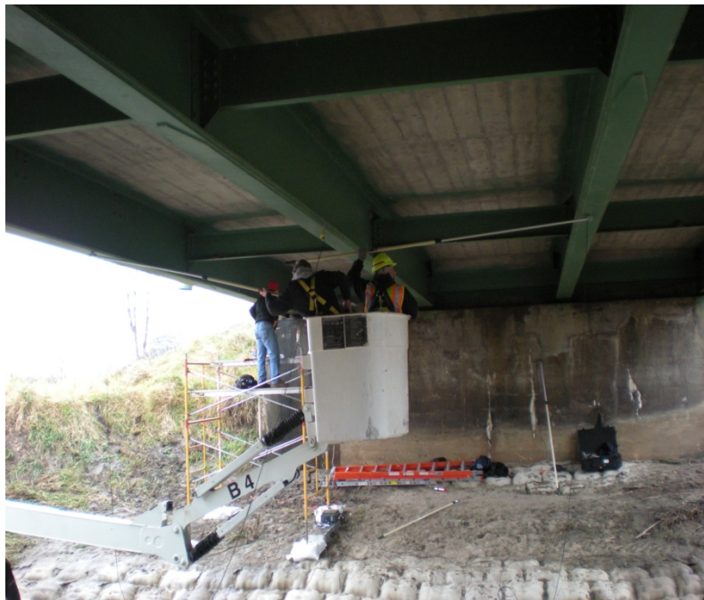
Figure 4.7 Snooper truck and long poles used to access the bottom flange of each beam
