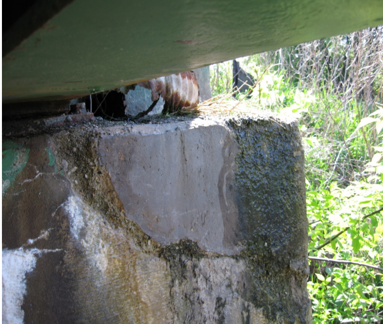
Figure 4.43 Large crack in the northeast abutment wall beneath beam 4
