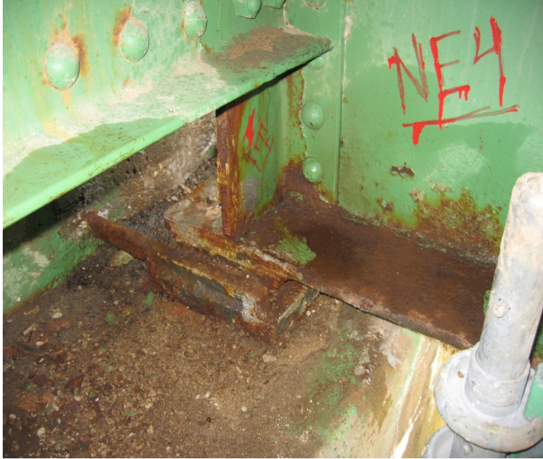
Figure 4.46 Forced vibration response measurement of northeast end and boundary condition of beam 4 with noticeable deterioration of the bottom flange
