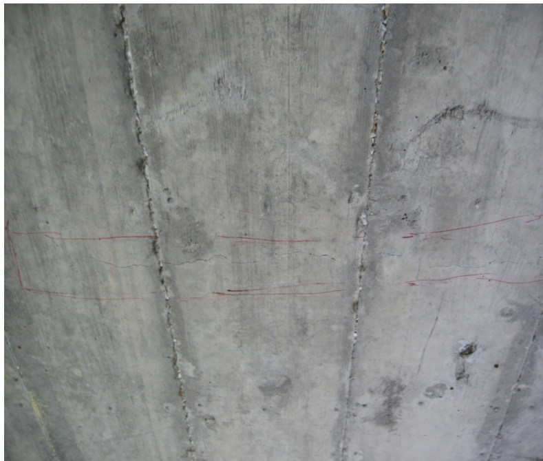
Figure 4.39 Lateral surface crack in concrete deck near midspan of bridge
