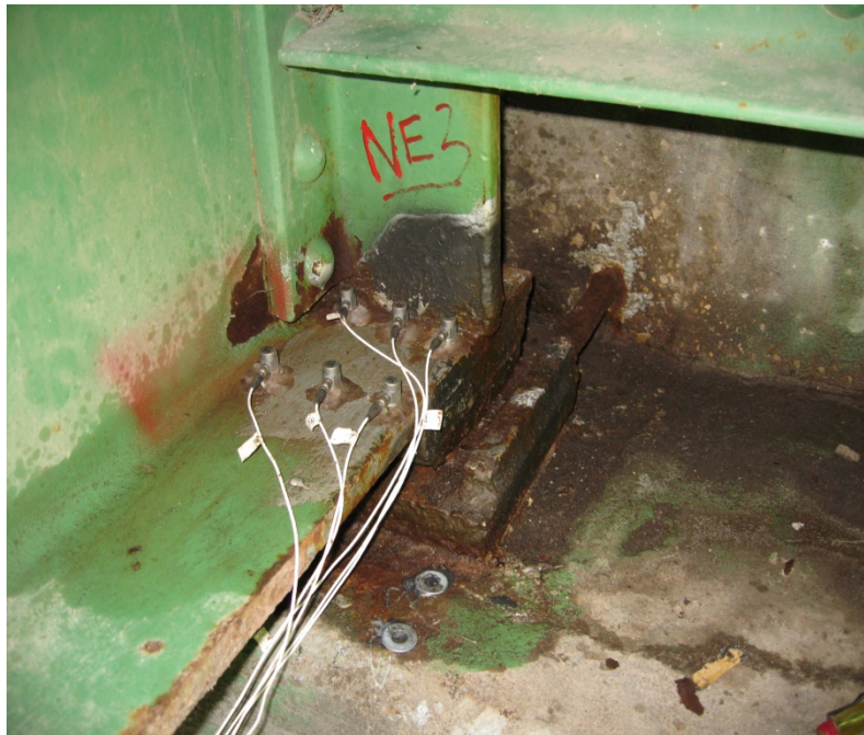
Figure 4.45 Forced vibration response measurement of northeast end and boundary condition of beam 3
