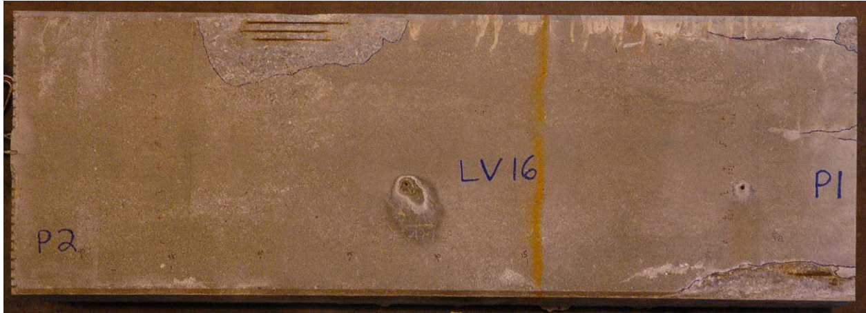
Figure 3-7: Bottom Flange Crack and Spall Condition Span 2 Beam 16
