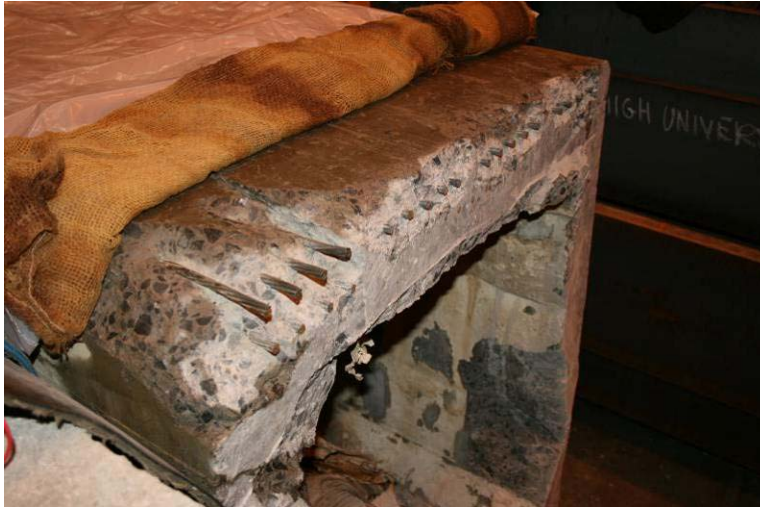
Figure 6-2: Exposed Strands at Sectioned Face of Beam
