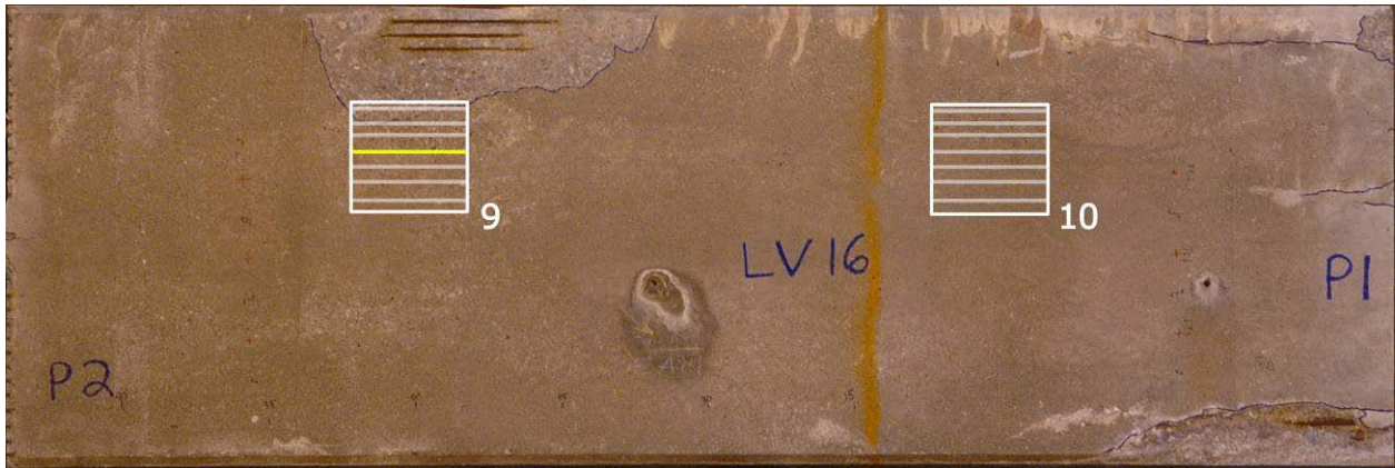
Figure 5-14: Location of 2 nd Layer Punchouts on Beam LV16
