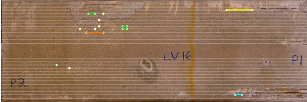
Figure 5-6: Damage Profile for Lakeview Drive Bridge Beam 16
