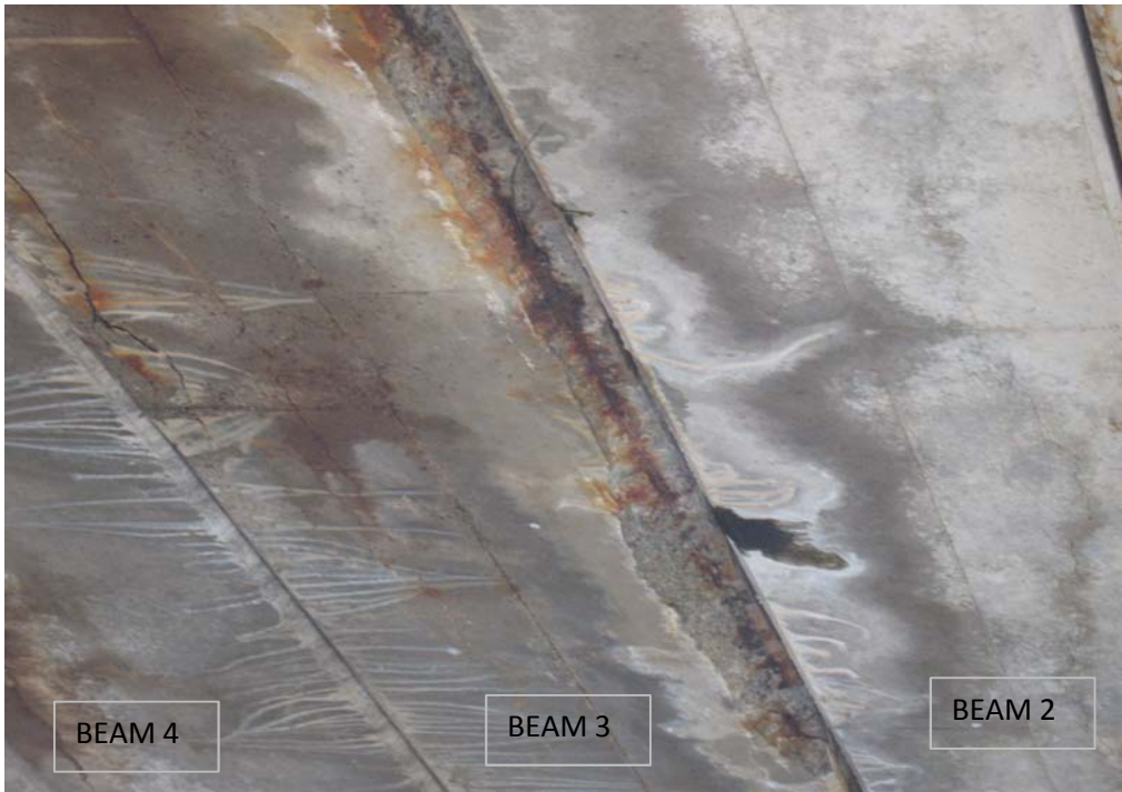
Figure 3 Underside of Beam 3 at mid-span, Looking back. Exposed strand on Beam 3 and longitudinal cracks.
