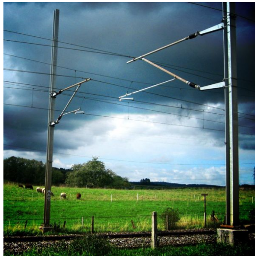
Figure 4 Swiss Federal Railways overhead lines
