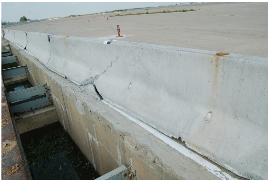
Figure 25. System Damage, Test No. NYTCB-5
