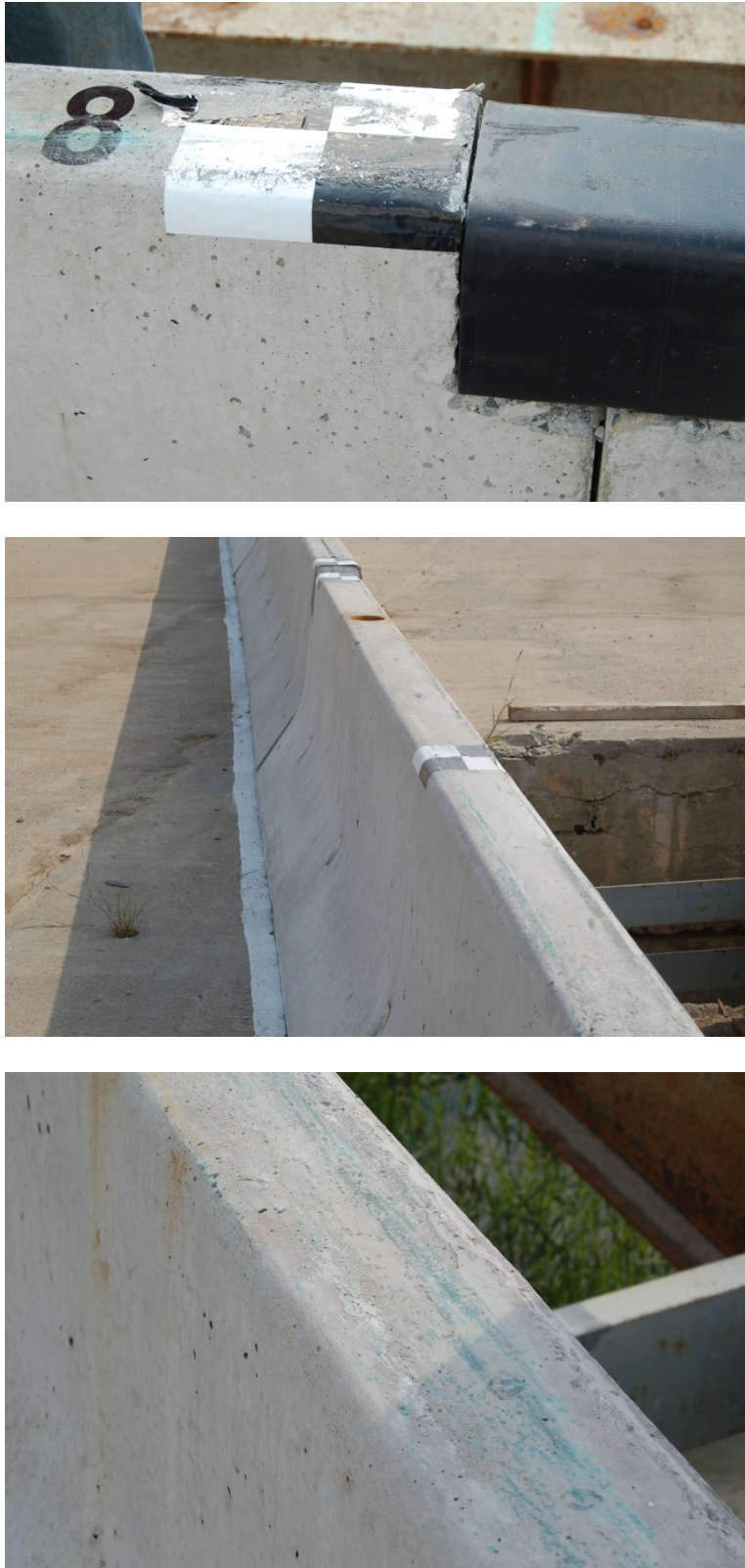
Figure 31. Barrier No. 8 Damage, Test No. NYTCB-5
