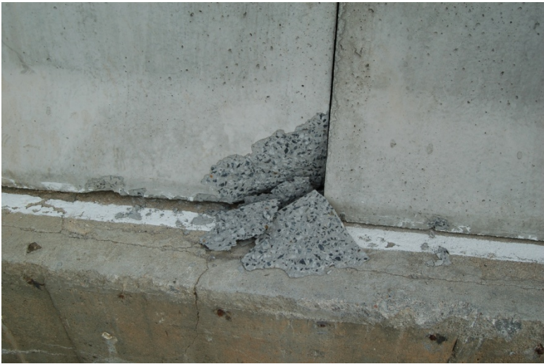
Figure 29. Barrier No. 5 Damage, Test No. NYTCB-5
