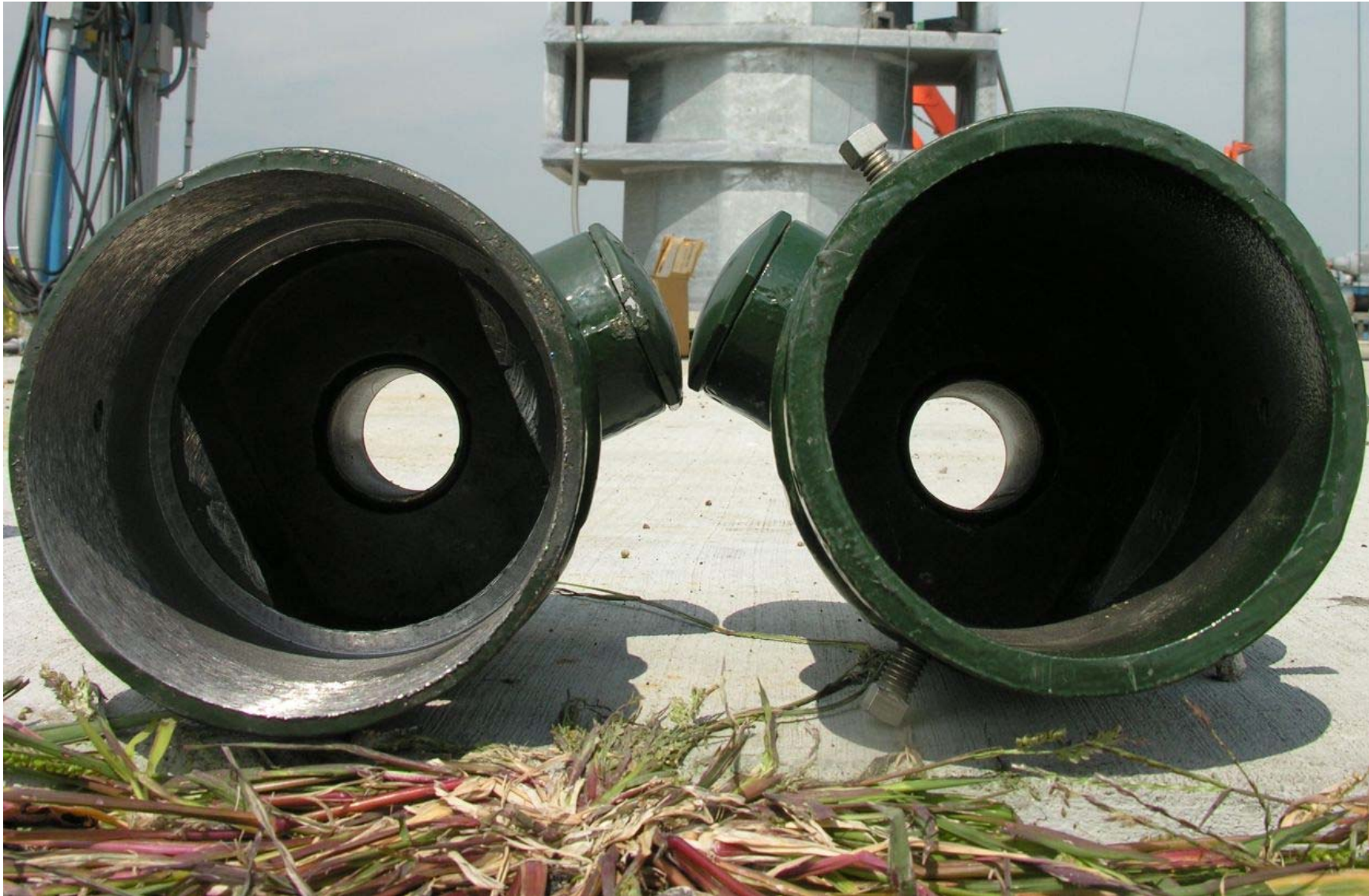
Figure 26. Left – Reduced Bracket Thickness, Right – Original Bracket Thickness
