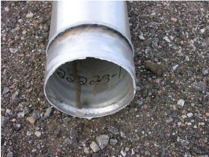
Figure 35. System Damage - Bottom Piece of Pole and Internal Sleeve, Test No. NYPP-1
