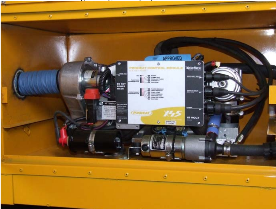
Figure 9 - Proheat X45 heater has been installed in the retrofitted compartment
