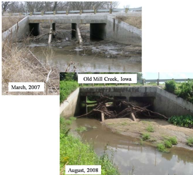
Figure 1-1 Typical sedimentation pattern at a culvert in Iowa
