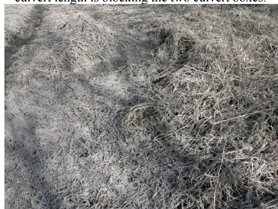
Mud trapped in the grass – observations made soon after a storm event passed through the culvert
