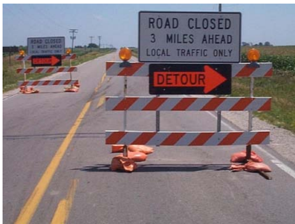
Figure 11. Typical Road Closure
