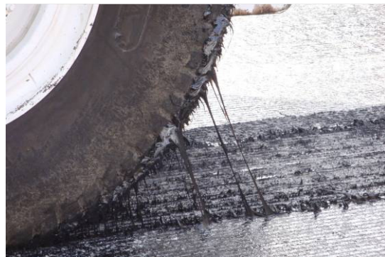
Figure 17. Bare streak left after PG asphalt tack picked up by Shuttle Buggy tire.
