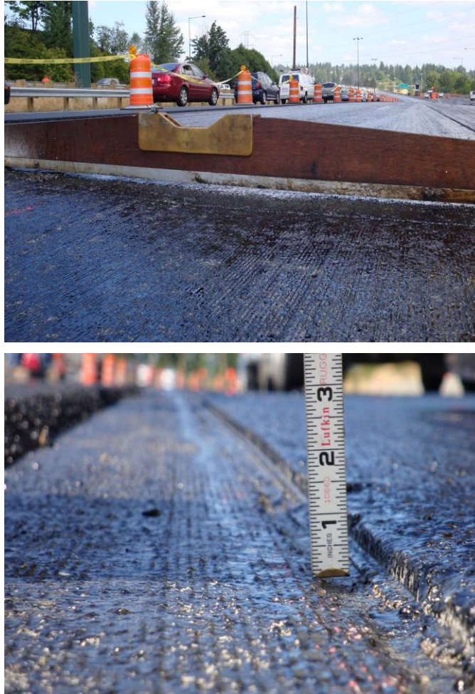
Amount of rutting present after milling
