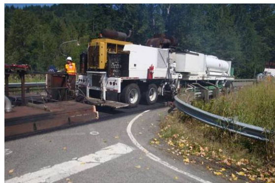
Figure 5. Right rear of unit A and towed trailer with heater.
