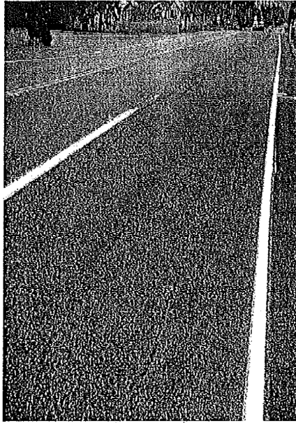
Photo 3 (~MP 4.8): Low to medium severity transverse & longitudinal reflective cracking.
