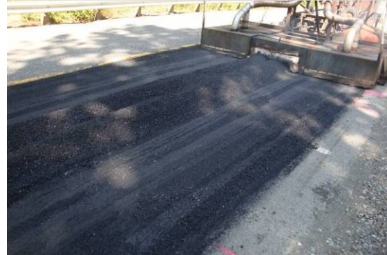
Figure 7. Milled HMA behind unit A is windrowed into the center of the lane.
