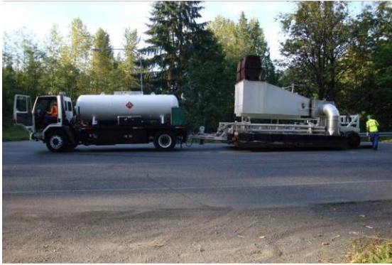
Figure 2. Preheater unit consisting of a propane truck and trailer with propane fired heaters.
