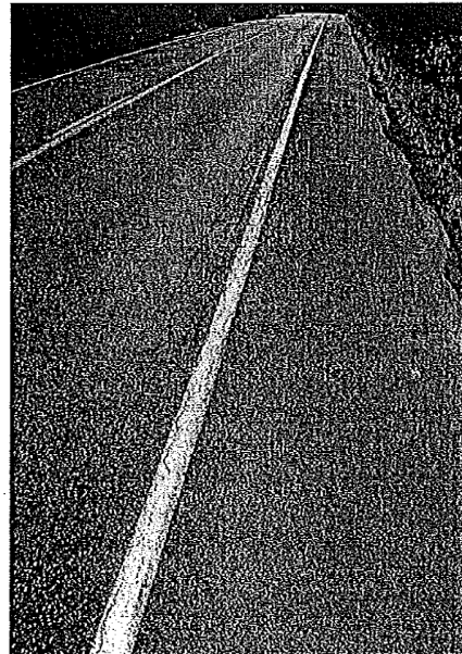
Photo 6 (~MP 14.27): Medium to high severity alligator cracking along the fog line and shoulder on WB lane.
