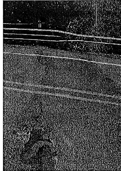
Photo 8 (~MP 17.65): High severity alligator cracking and settlement that was patched with HMA by maintenance at both ends of the bridge #542/21.
