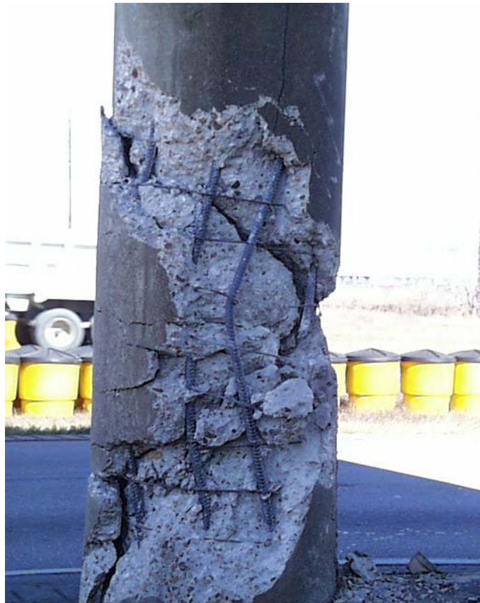
Figure 3.1. Typical Failure Mechanism in Bridge Pier from Large Truck Collision.
