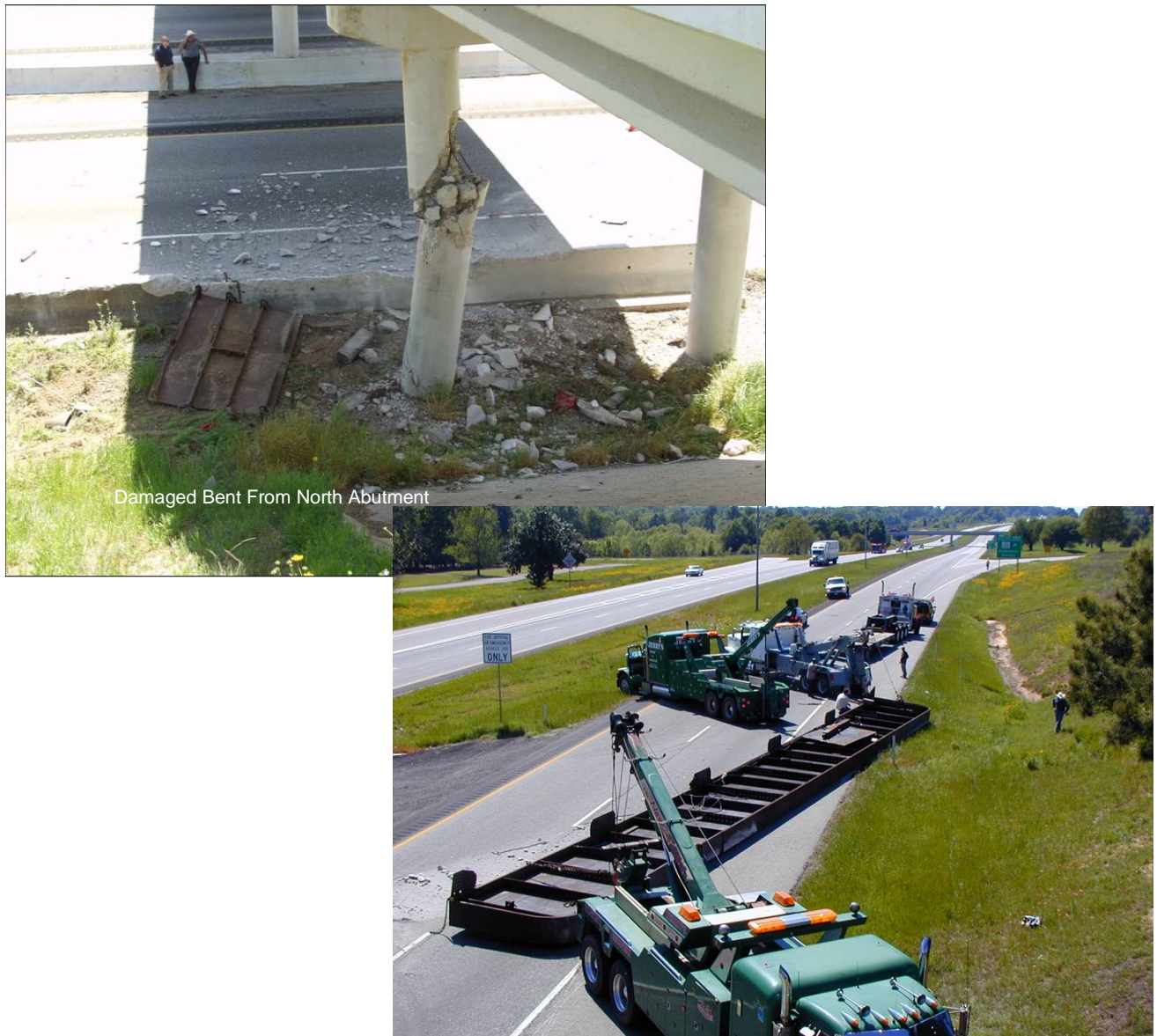
Figure 2.5. Truck Accident – FM 2207 Bridge over IH-20, Tyler, Texas.
