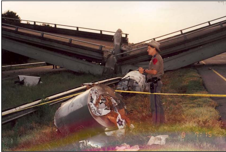
Figure 2.1. Truck Accident FM 2110 Bridge over IH-30, Texarkana, Texas.
