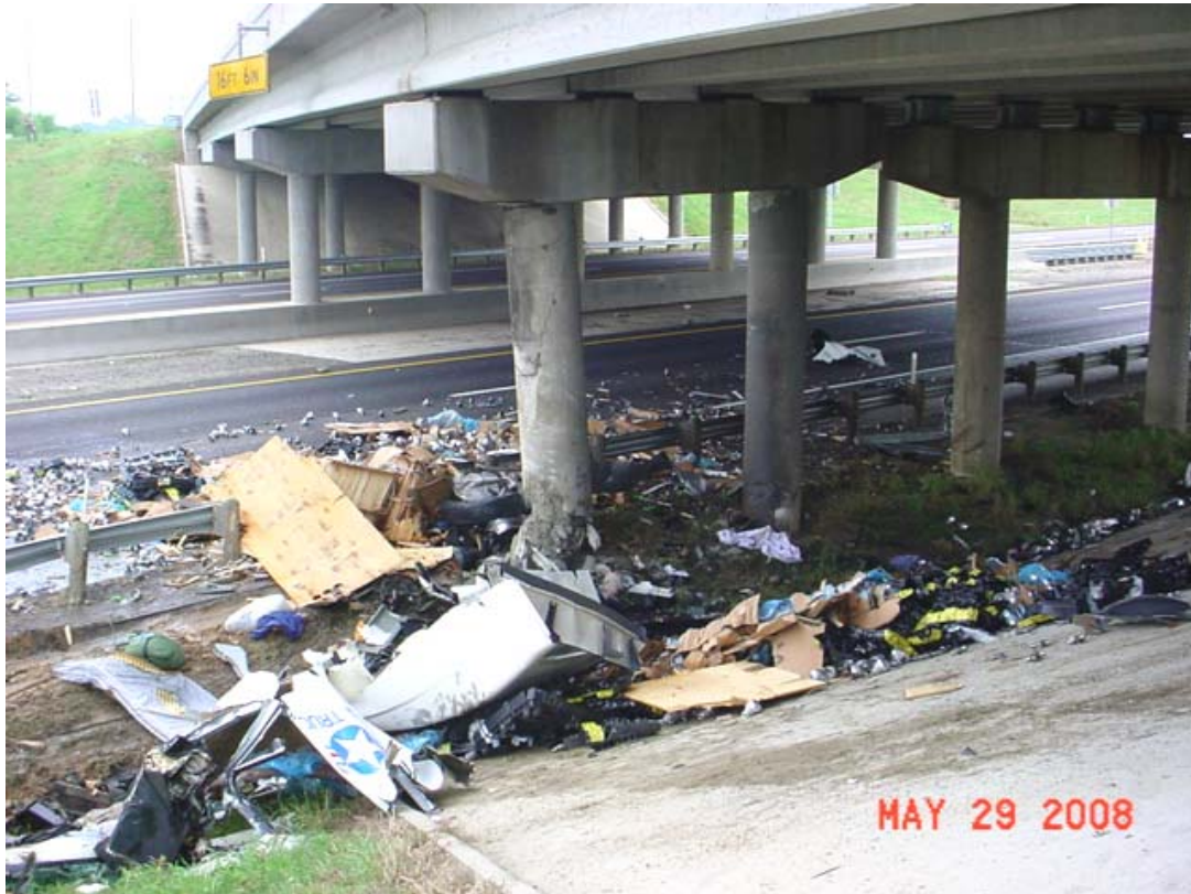
Figure 2.11. Truck Accident – FM 1401 Bridge over IH-30, Mount Pleasant, Texas.
