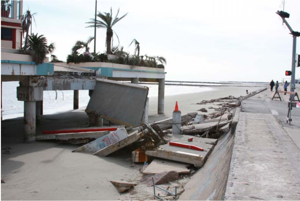
Figure 27. Damage to the Entrance Bridge to Flagship Hotel, Galveston.
