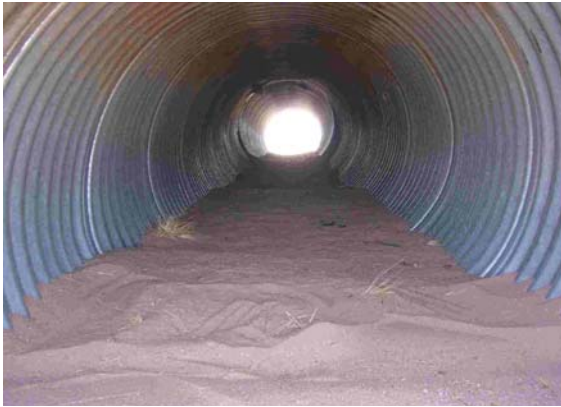
Figure 3. Soil from the site distributed through the 36-in diameter culvert without skylights.
