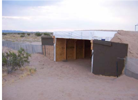
Figure 4. Entrance of the 4-ft by 8-ft box culvert with a skylight (upper right) and headwalls (dark brown).
