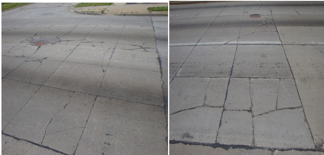
Figure 18. Condition of Fond Du Lac Avenue (2009)
