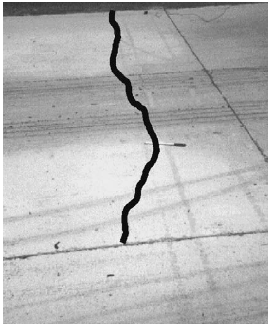
Figure 6. Mid-Slab Cracking (Rasmussen et al. 2002)
