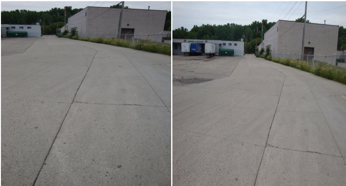
Figure 23. Condition of State Street (2009)
