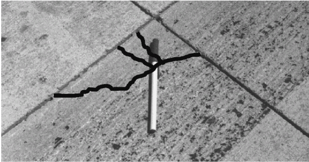
Figure 11. Spalling (Rasmussen et al. 2002)
