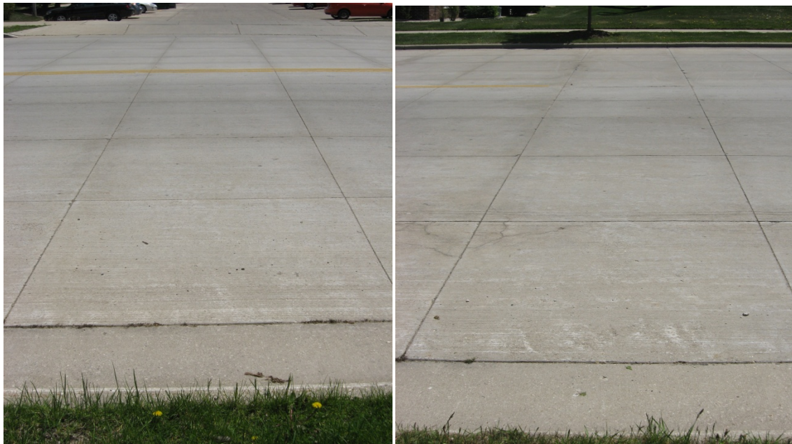
Figure 22. Condition of North 39 th Avenue (2008)
