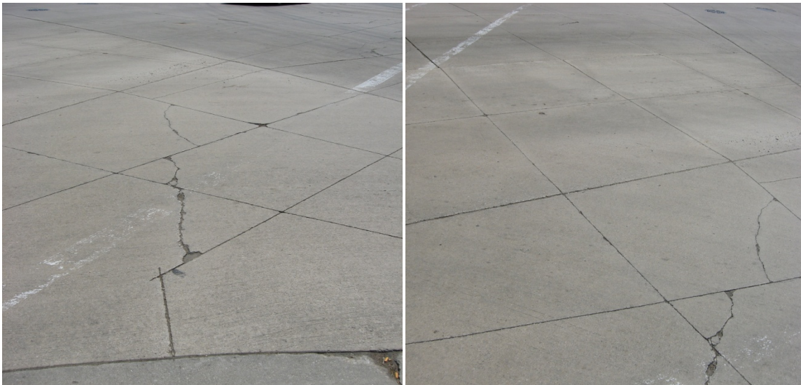
Figure 29. Condition of Washington Street and 22 nd Street Intersection (2008)
