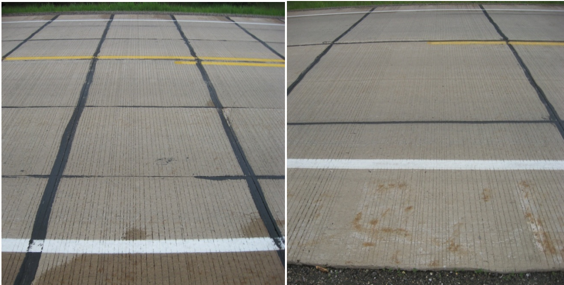
Figure 27. Condition of STH 82 (2008)
