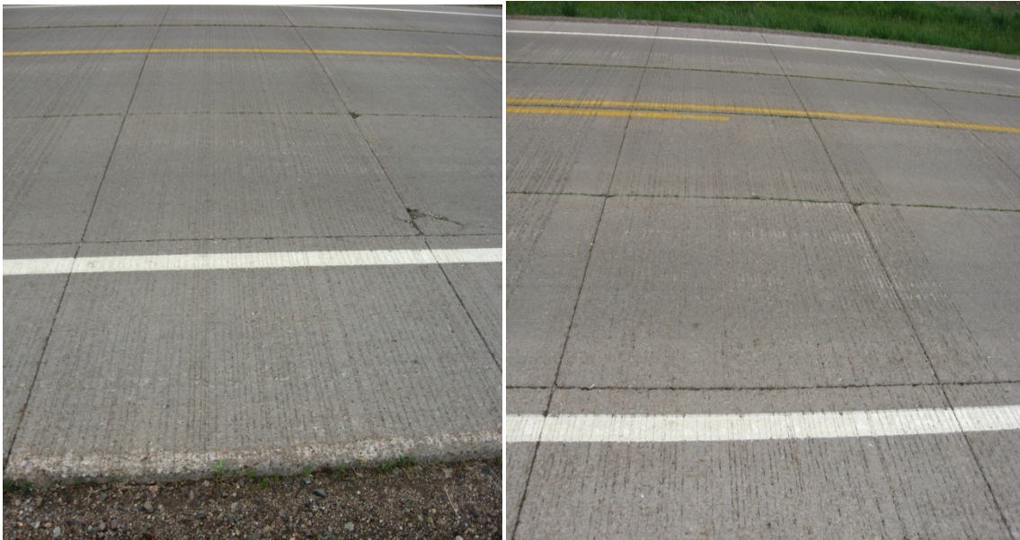
Figure 28. Condition of STH 97 (2008)
