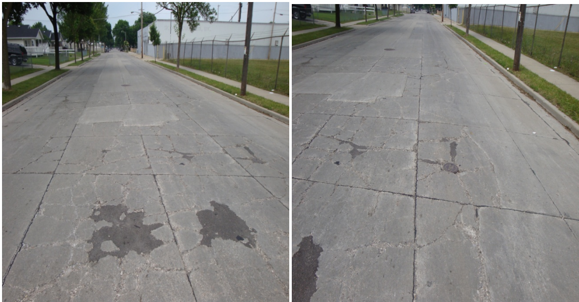
Figure 19. Condition of Galena Street (2009)
