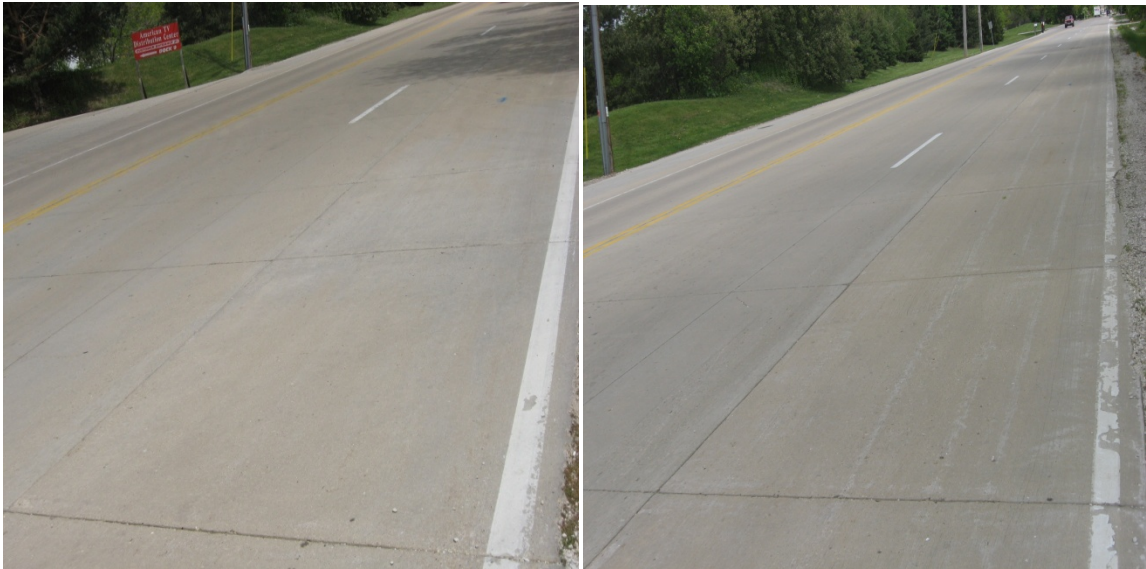
Figure 17. Condition of Duplainville Road (2008)
