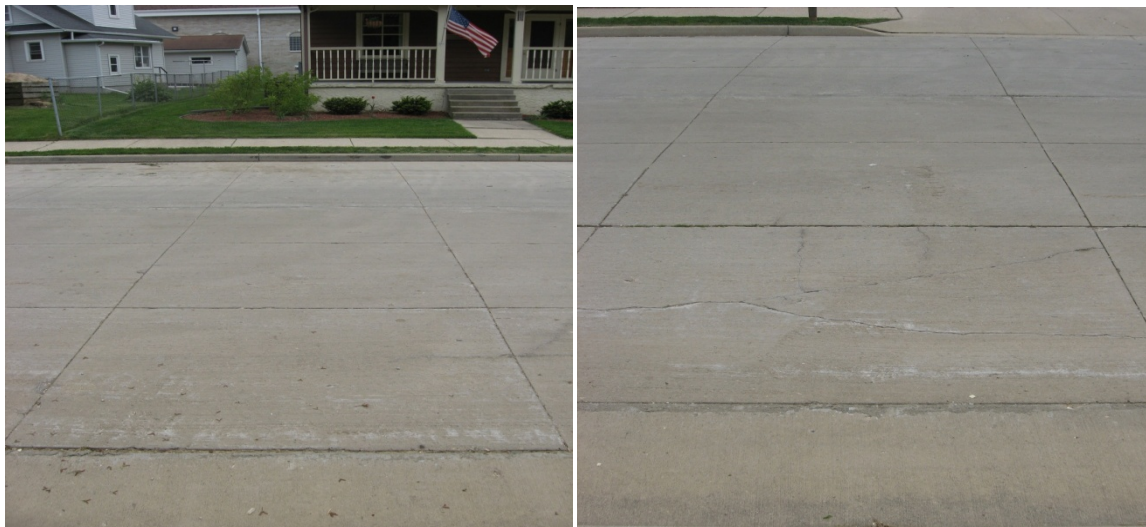
Figure 21. Condition of Lawndale Avenue (2008)
