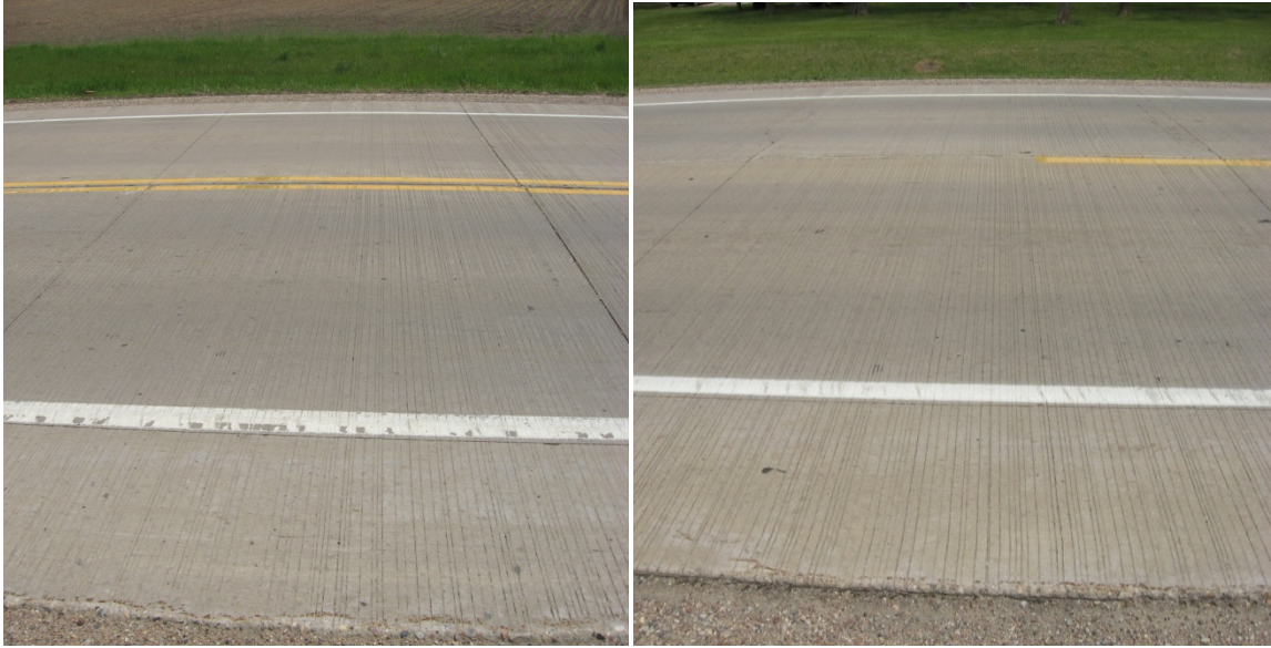
Figure 26. Condition of STH 54 (2008)
