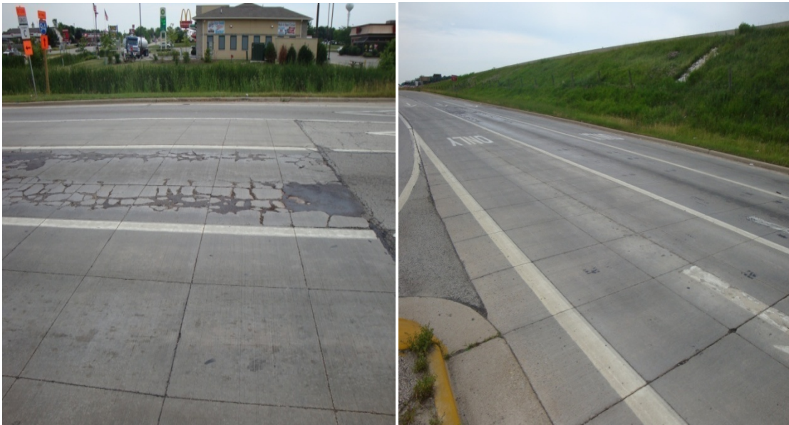
Figure 20. Condition of IH 94/STH 50 Ramp (2009)
