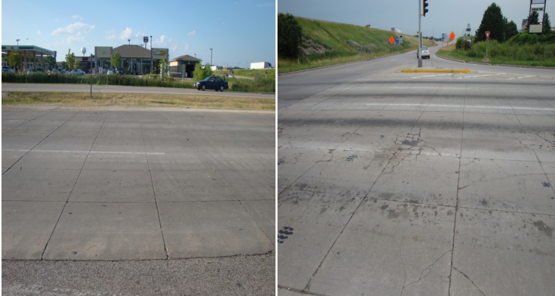
Figure 25. Condition of STH 50 (2009)
