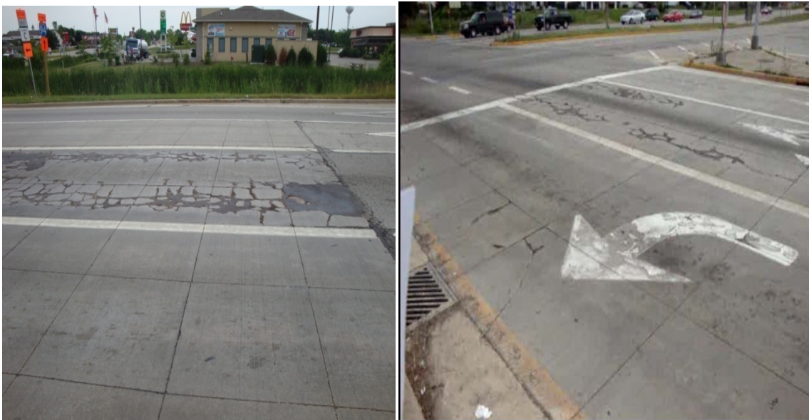
Figure 44. Localized Severe Distress at the Entrance (left) and Exit (right) End of IH94/USH50 Ramp
