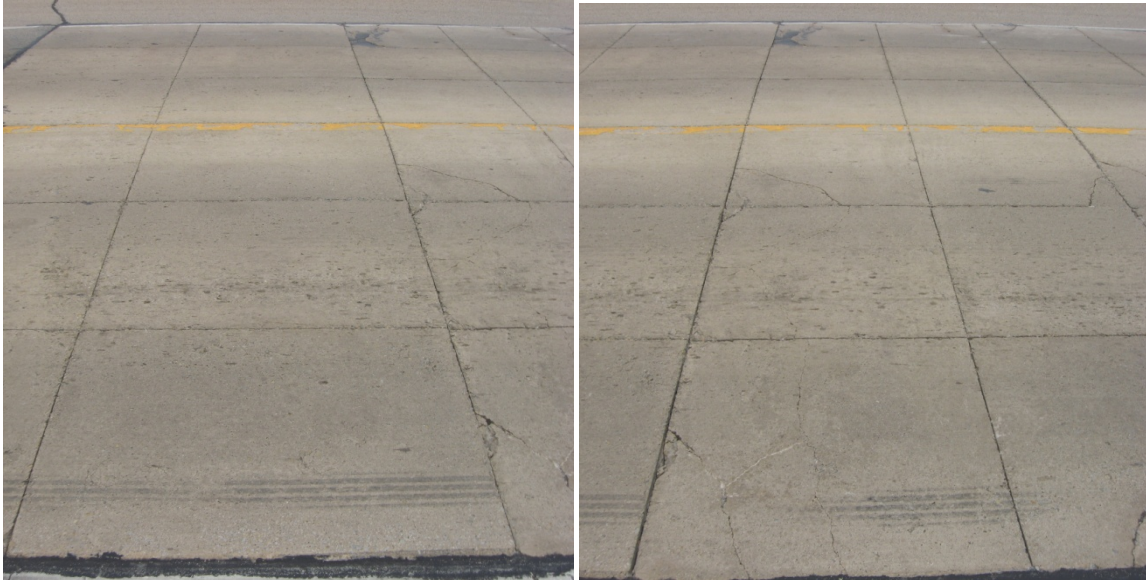
Figure 24. Condition of STH33 and CTH “A” (2008)
