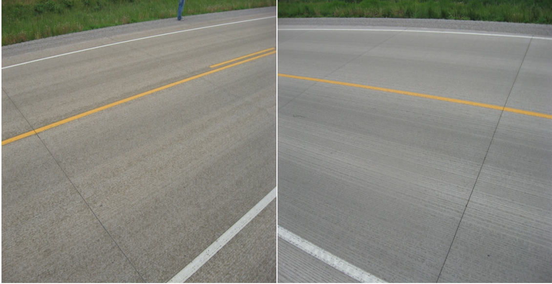
Figure 16. Condition of CTH “A” (2008)
