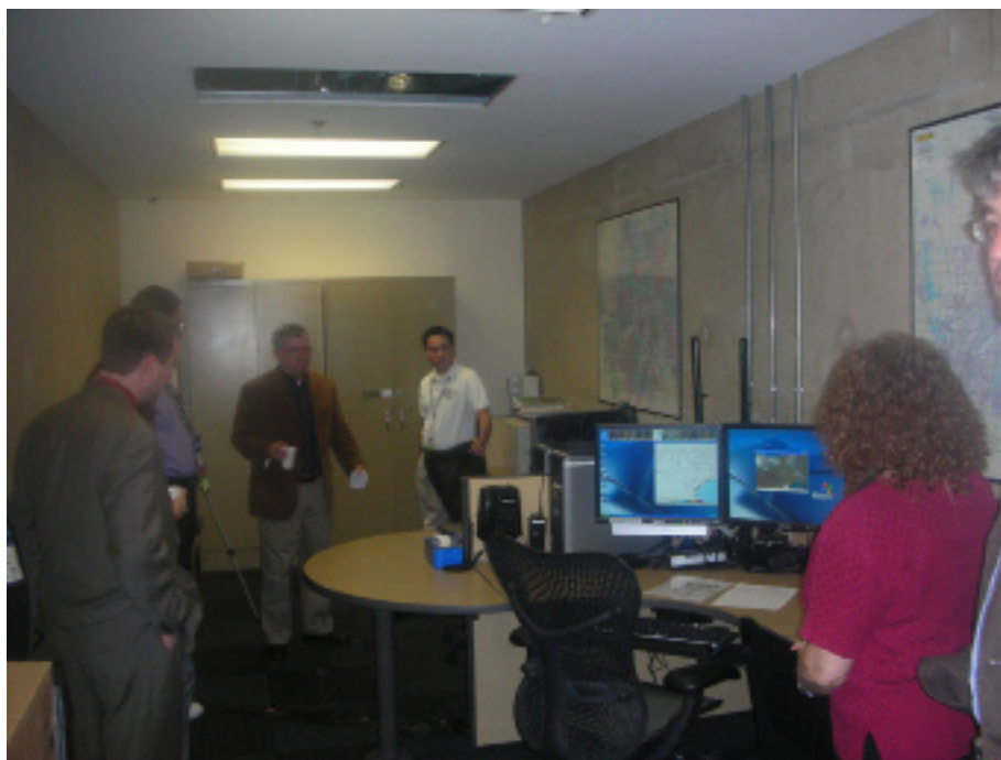
Figure 13 Dallas EOC Radio Room
