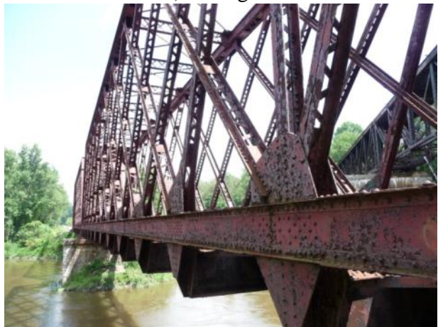
d) Left side (span 1)
