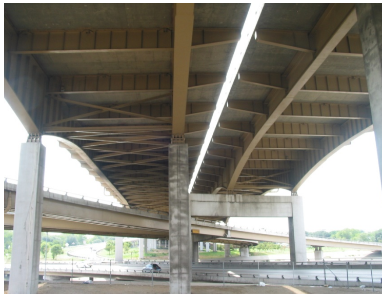
Figure 5.2: Intersection of IH 30
