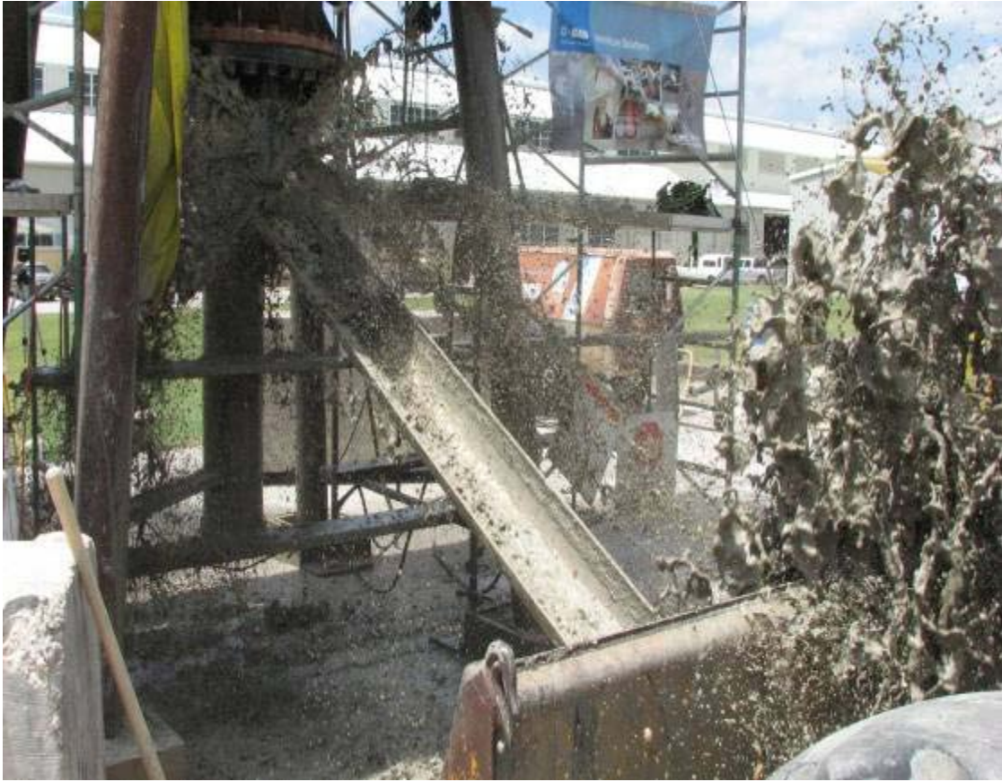
Figure 2.2.19 – Water Gushing out of rocket during evacuation of concrete poured under wet condition
