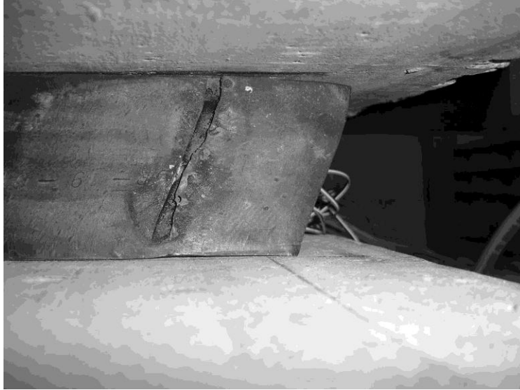
Figure 5.67 – Example of Observed Transverse Top Uplift
