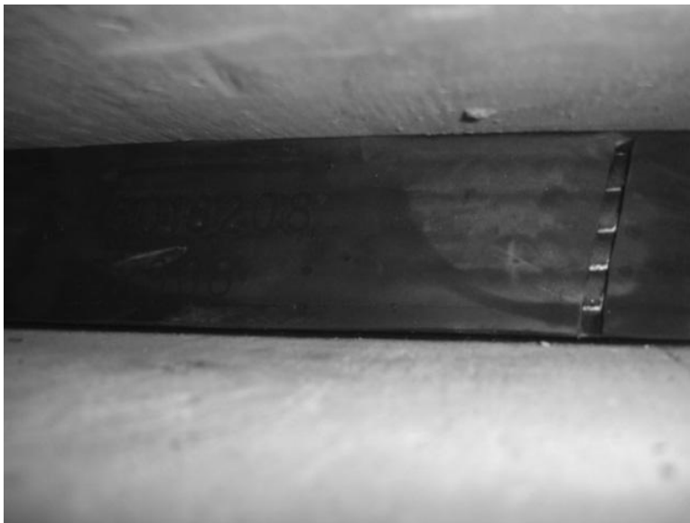
Figure 5.77 – Exposure of Shims
