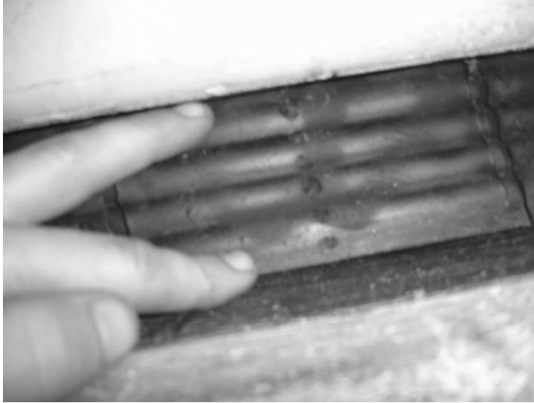
Figure 5.75 – Tension Debonding at Shims
