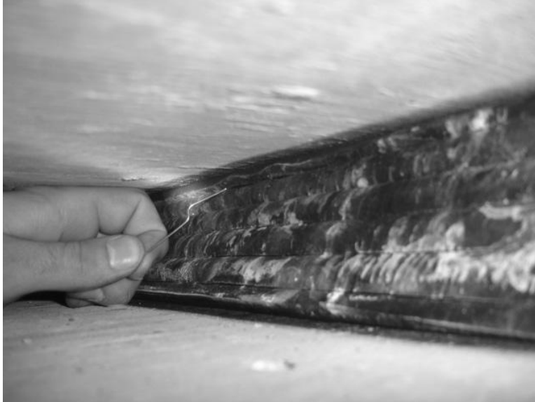
Figure 5.76 – Delamination of Elastomer
