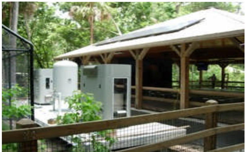
A 5 kW photovoltaic array on the roof of this pavilion runs an electrolyzer that generates hydrogen fuel for a Hydrogenics PEM fuel cell at Homosassa Wildlife Park, Homosassa, Florida.
