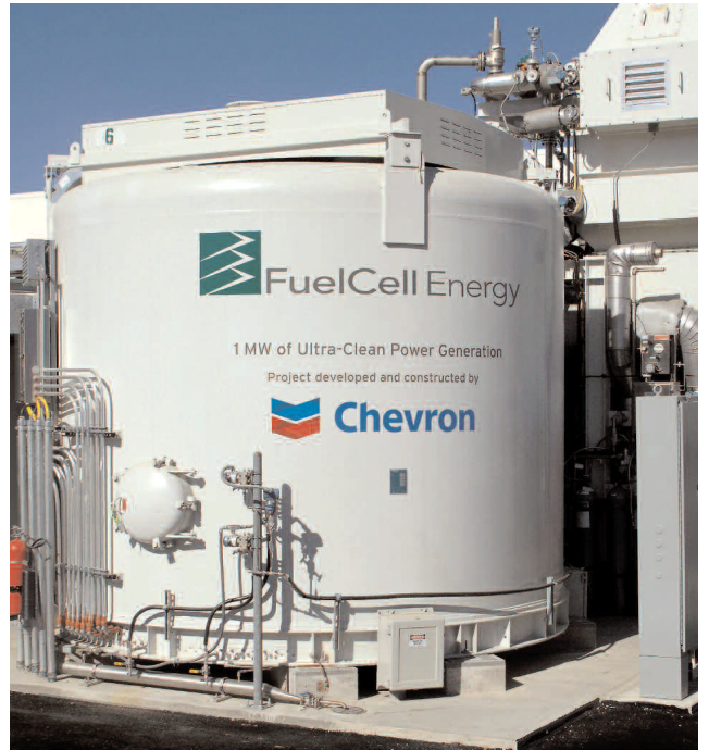
Four 250 kW units from FuelCell Energy provide 90% of the Santa Rita Jail's base load power. The project used funding from the California Public Utilities Commission's Self Generation Incentive Program.
