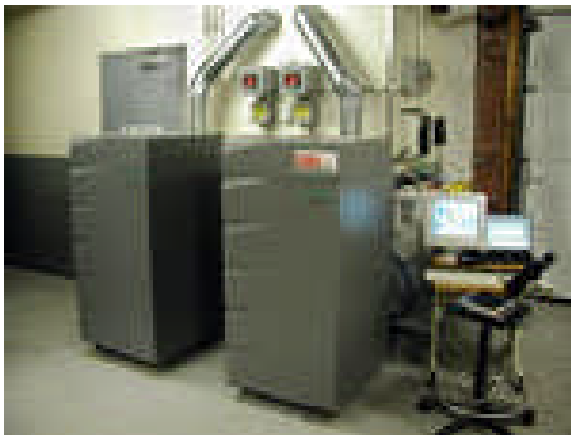
The US Coast Guard Aid to Navigation Team maintenance facility in Bristol, Rhode Island hosted a Department of Defense Residential PEM Fuel Cell Demonstration Project installation.
