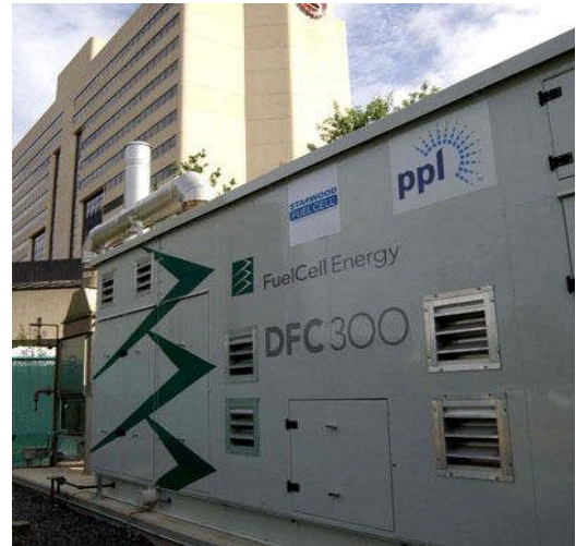
The Sheraton Hotel in Edison, New Jersey uses a 250 kW molten carbonate fuel cell from FuelCell Energy. The fuel cell provides 25% of the hotel's electric and hot water needs.
