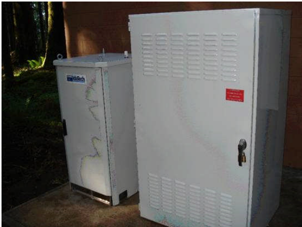
This IdaTech PEM fuel cell system provides back-up power to the Oregon State Police emergency response transmitters. The fuel cell replaces a diesel generator.
