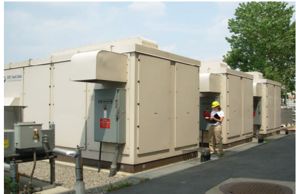
The Hunts Point Waste Water Treatment Plant, in the Bronx, New York, uses three 200 kW units from UTC Power that operate in parallel with the grid.
