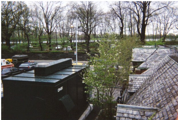
New York Police Department in Central Park uses a 200 kW phosphoric acid fuel cell from UTC Power that operates independently from the grid. During a major city-wide power outage in 2003, the station was unaware of the situation because the fuel cell continued to supply electricity to the building.
