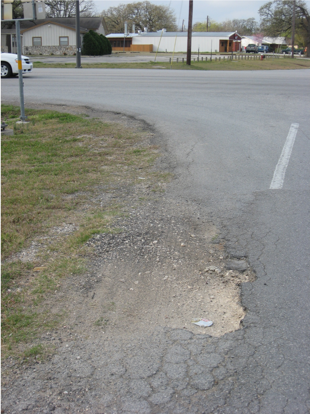
Figure 1. Pavement Damage from Trucks Tracking Off Pavement at a Short Corner Radius.
