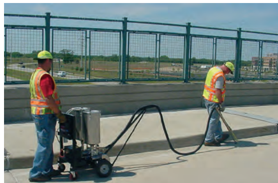
Report 2009-13 established best-practice guidelines for concrete deck and crack sealing on Minnesota's bridges.
