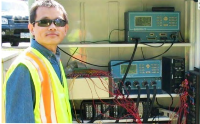
SMART-SIGNAL's data collection devices installed in a France Avenue signal controller cabinet received data from vehicle detection units and the traffic signal controller.
