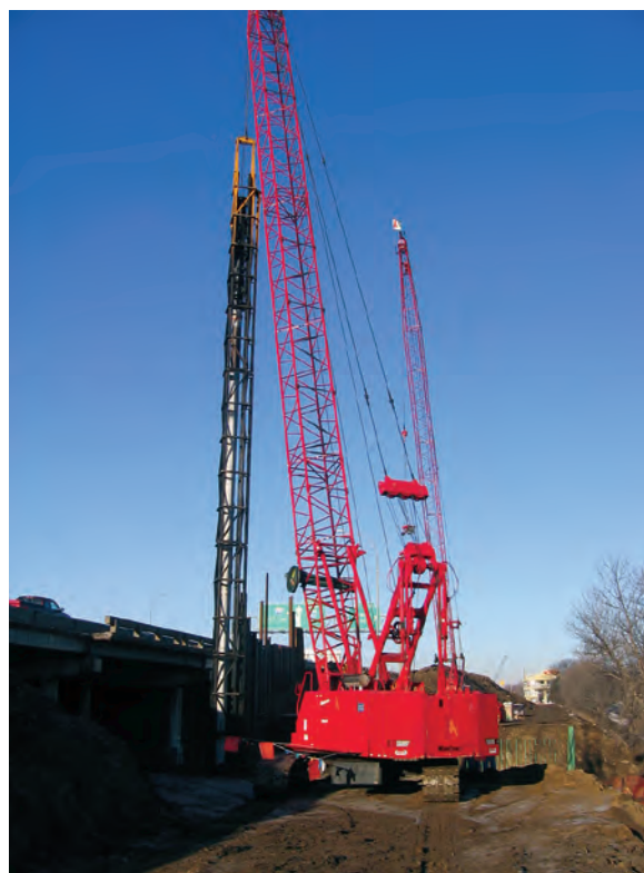
Mn/DOT funded research ( Reports 2009-37 and 2009-38 ) to improve the efficiency of pile driving operations, enabling construction crews to build safe foundations for bridges with less expense.
