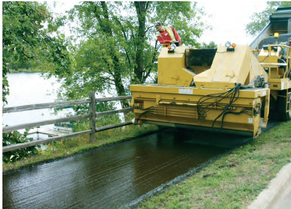
The LRRB-sponsored Report 2009-25 , Preventive Maintenance for Recreational Trails , describes how techniques designed for roadways such as chip sealing (pictured here) need to be modified for use on trails.
