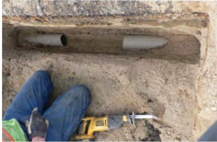
Researchers cut out sections of edge drain pipes to evaluate sediment composition.
